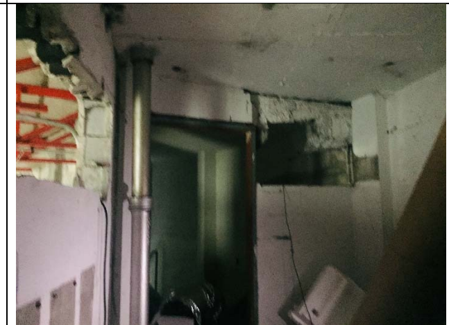
2022 – Mezzanine AHU Room
