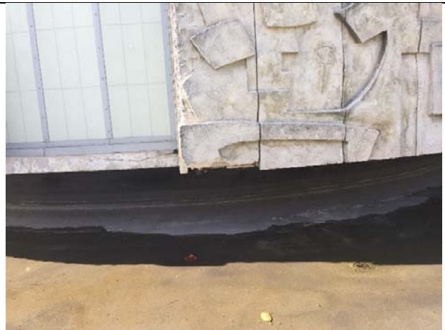
2022 – North window bottom panel damaged
