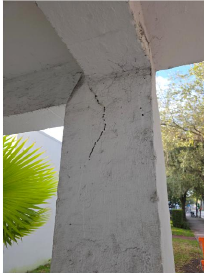
Spall and delaminated stucco and concrete present
