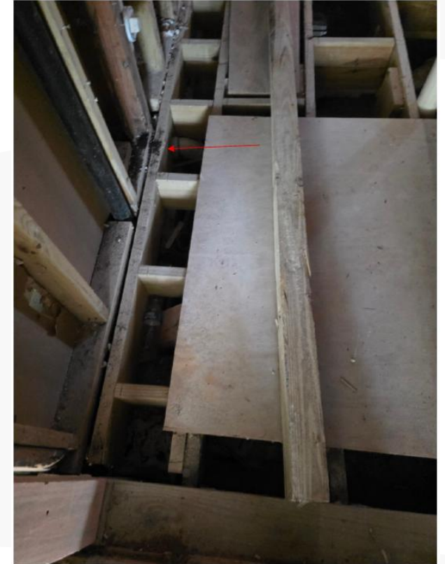
Termite dropping and stud damage
