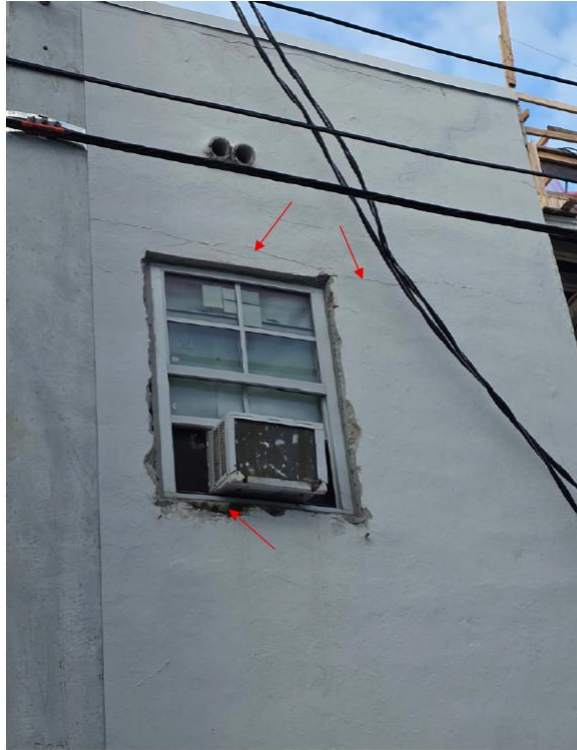
Spall and delaminated stucco and concrete present
