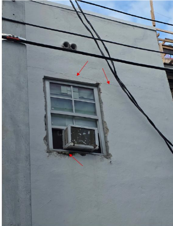
Spall and delaminated stucco and concrete present
