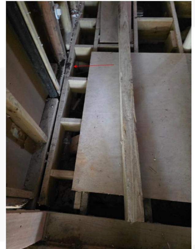
Termite dropping and stud damage
