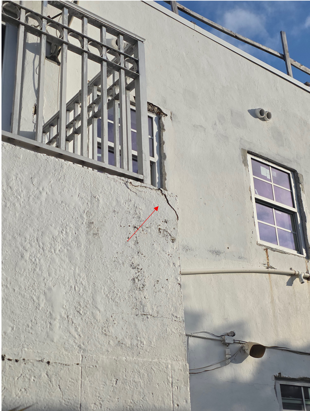
Spall and delaminated stucco and concrete present
