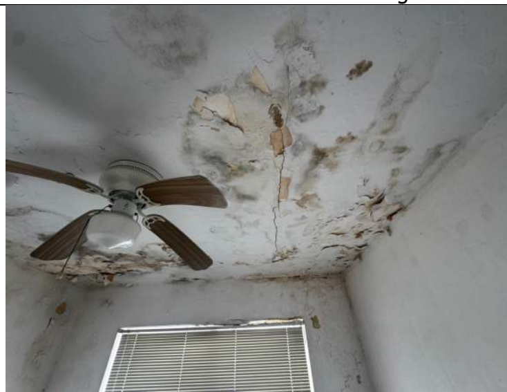
Roof moisture penetration damage
