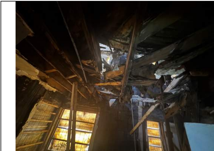
2 nd floor wood failure
