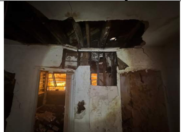
Wood Damage and failure
