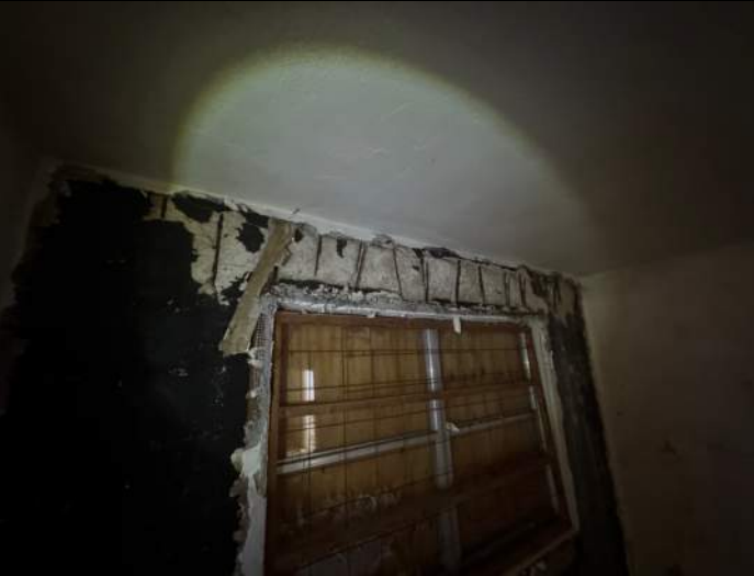
Concrete beam spalling and rebar corrosion
