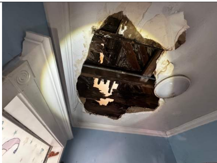
2 nd floor wood failure
