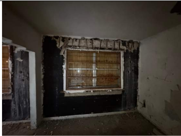
2 nd floor concrete beam damage
