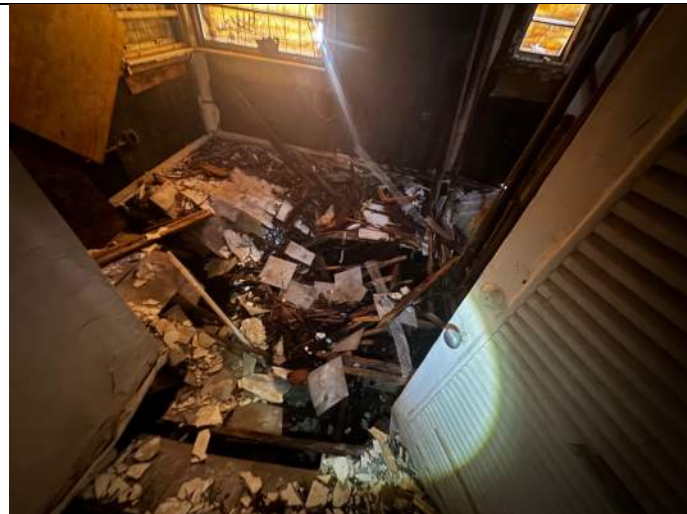
1 st floor wood failure
