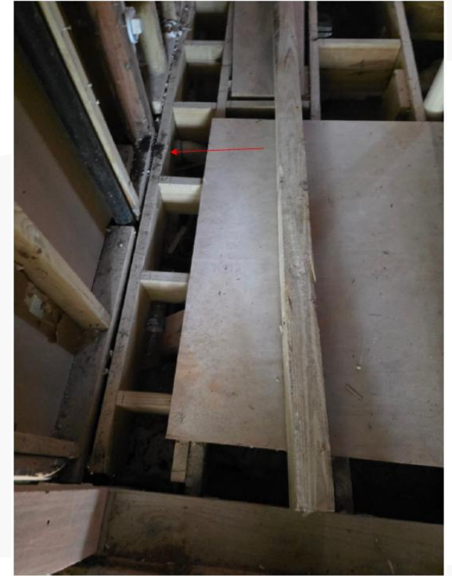
Termite dropping and stud damage
