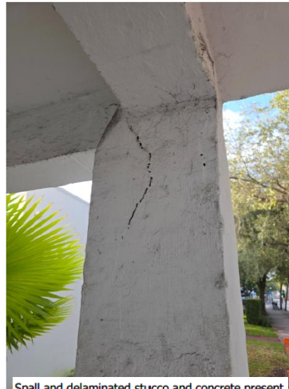
Spall and delaminated stucco and concrete present
