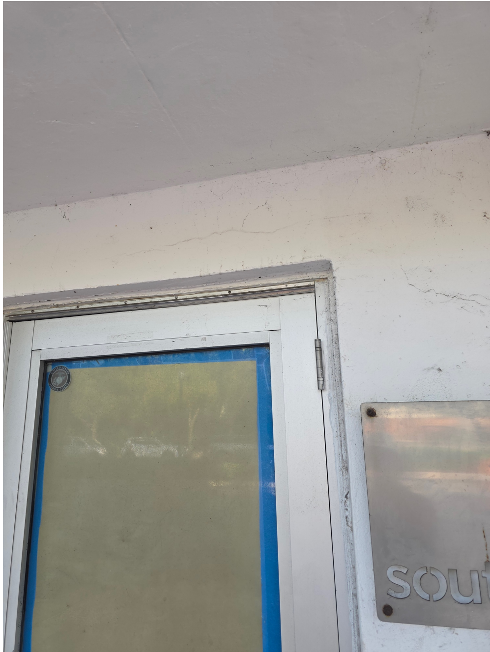
Spall and delaminated stucco and concrete present
