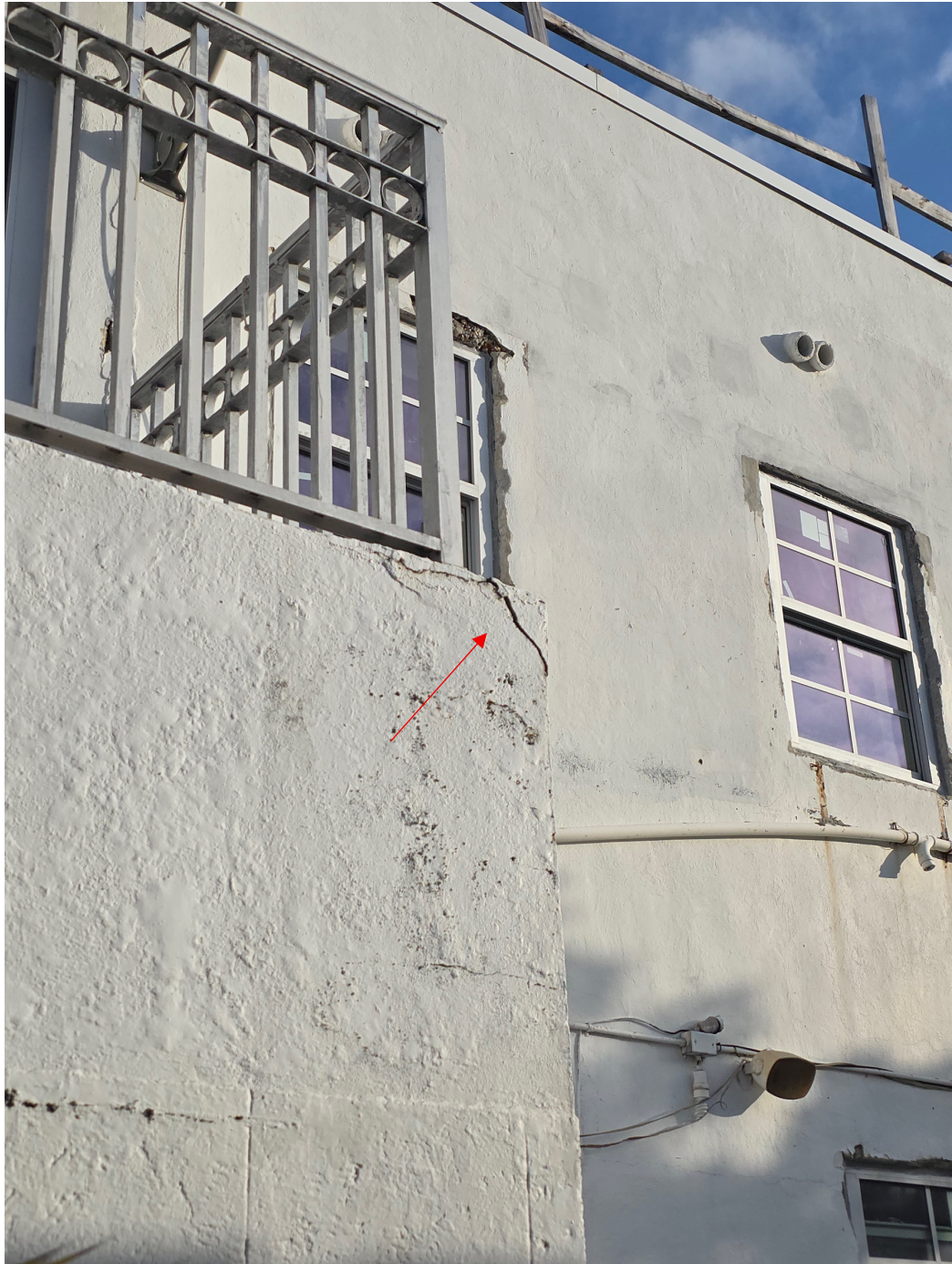
Spall and delaminated stucco and concrete present
