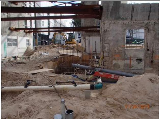
Carlton dewatering well point system
