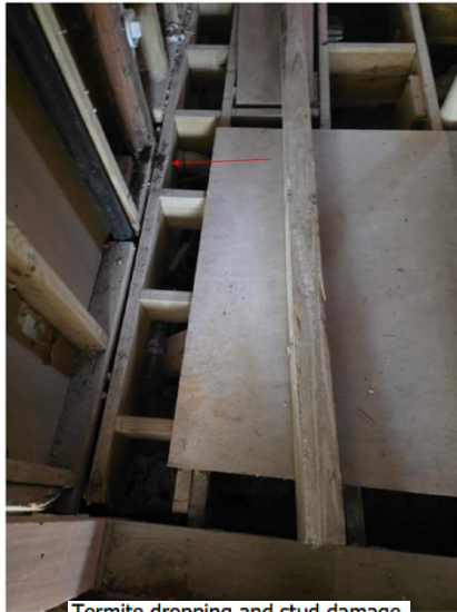
Termite droppings and stud damage
