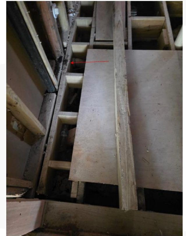
Termite dropping and stud damage
