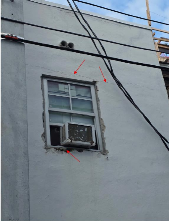
Spall and delaminated stucco and concrete present
