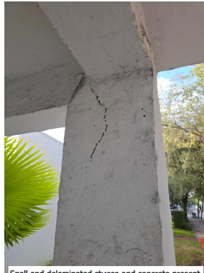
Spall and delaminated stucco and concrete present
