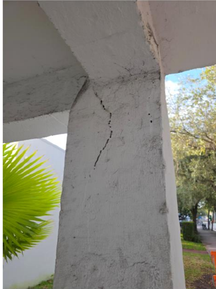
Spall and delaminated stucco and concrete present
