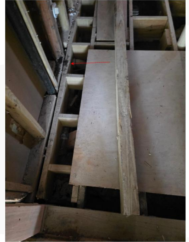
Termite dropping and stud damage
