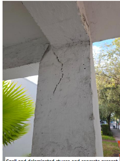
Spall and delaminated stucco and concrete present
