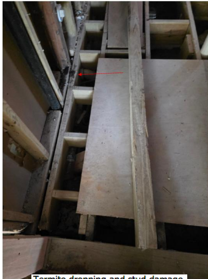
Termite dropping and stud damage
