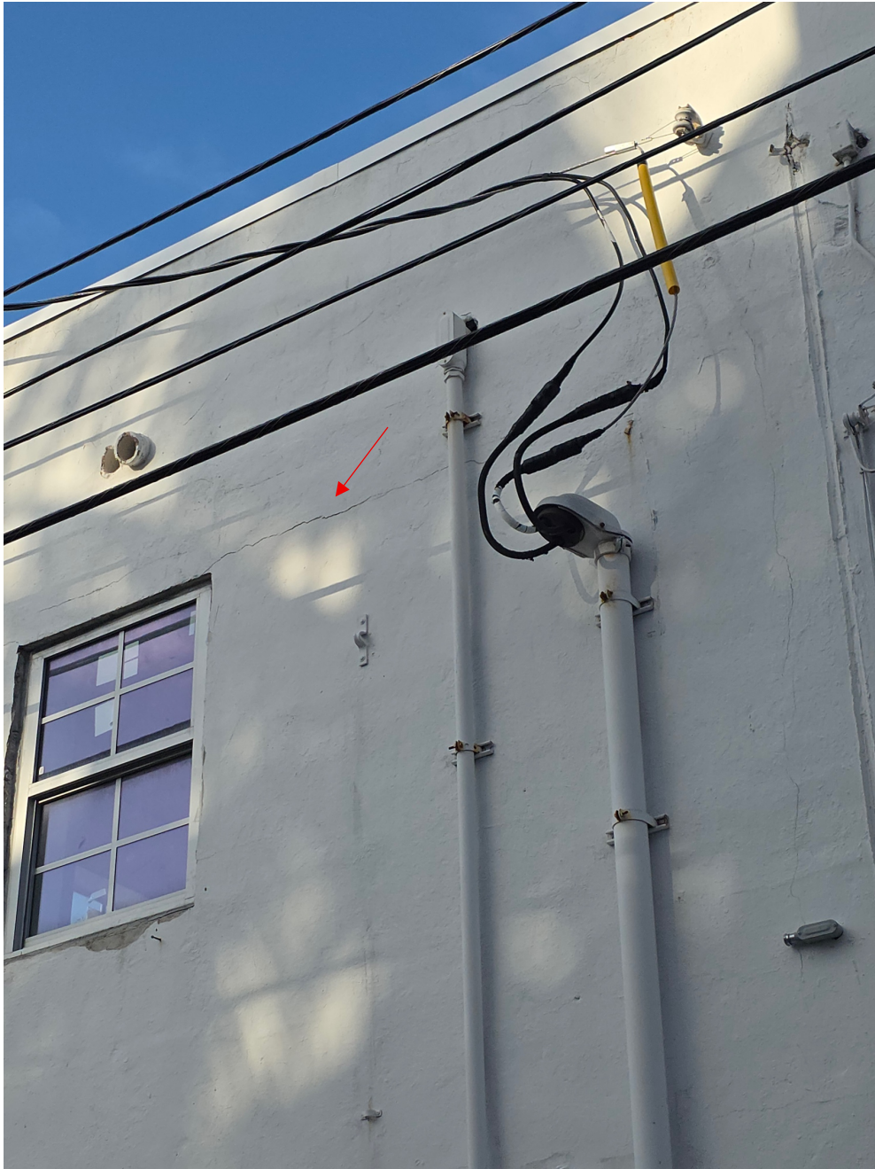
Spall and delaminated stucco and concrete present
