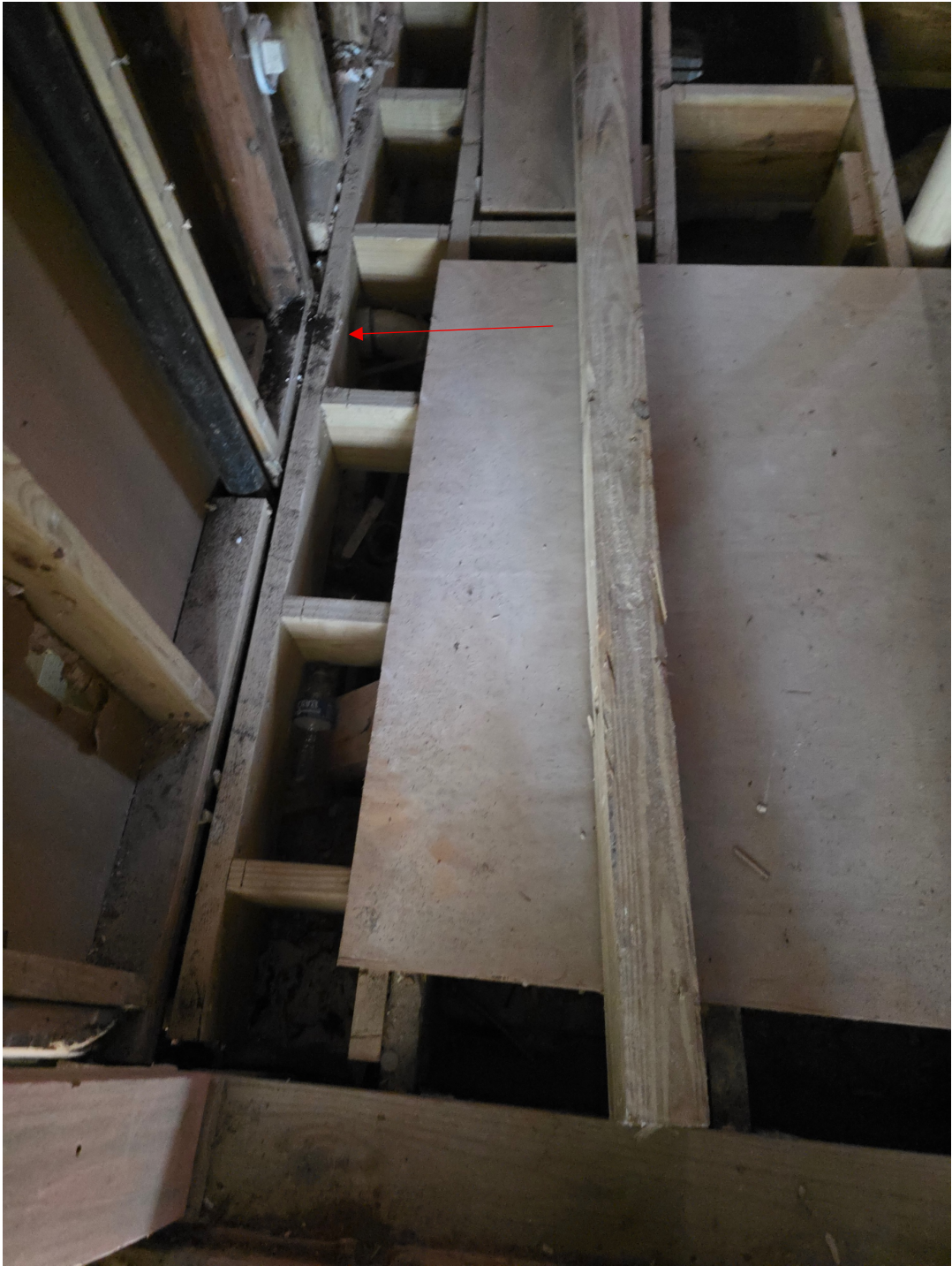
Termite dropping and stud damage
