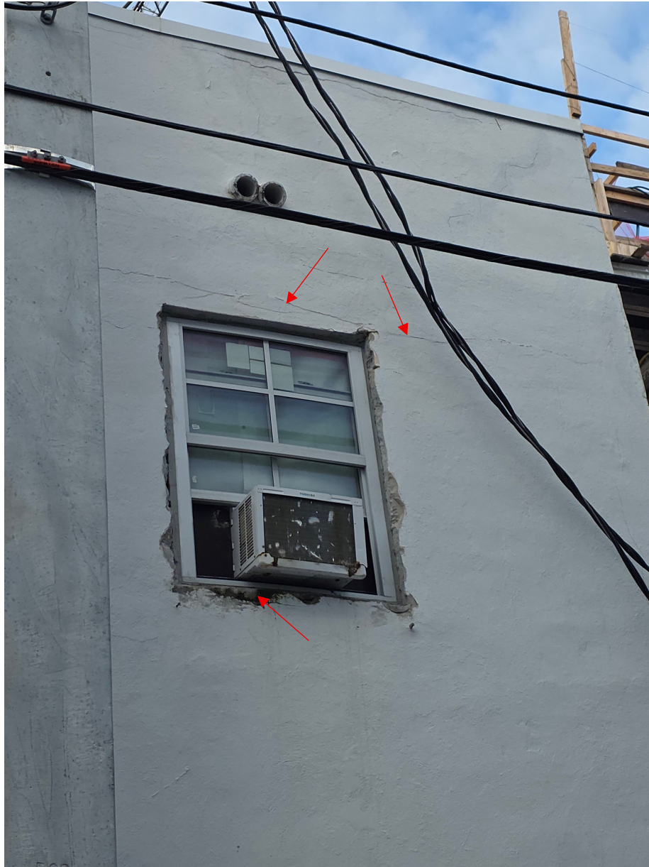
Spall and delaminated stucco and concrete present
