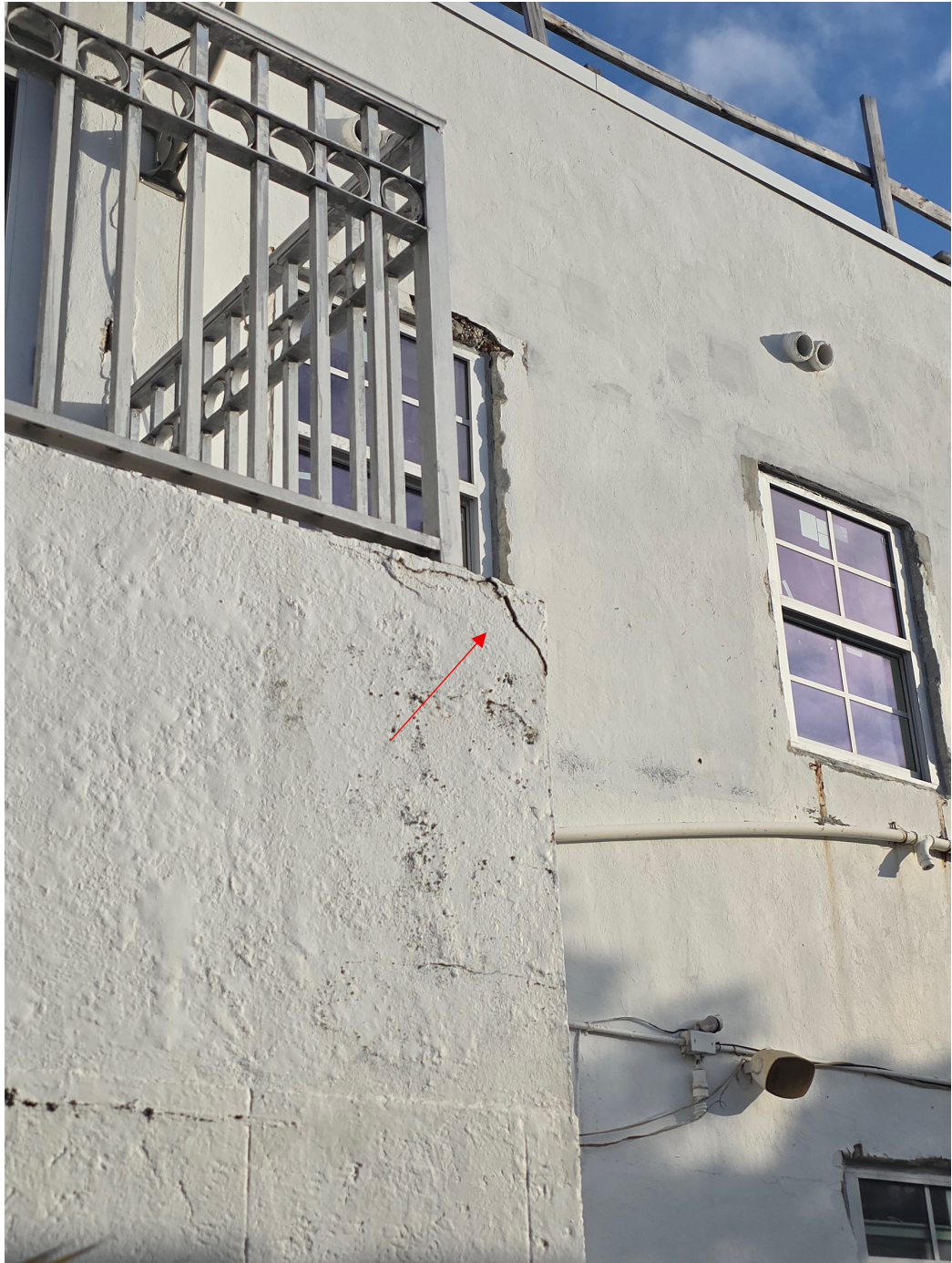
Spall and delaminated stucco and concrete present
