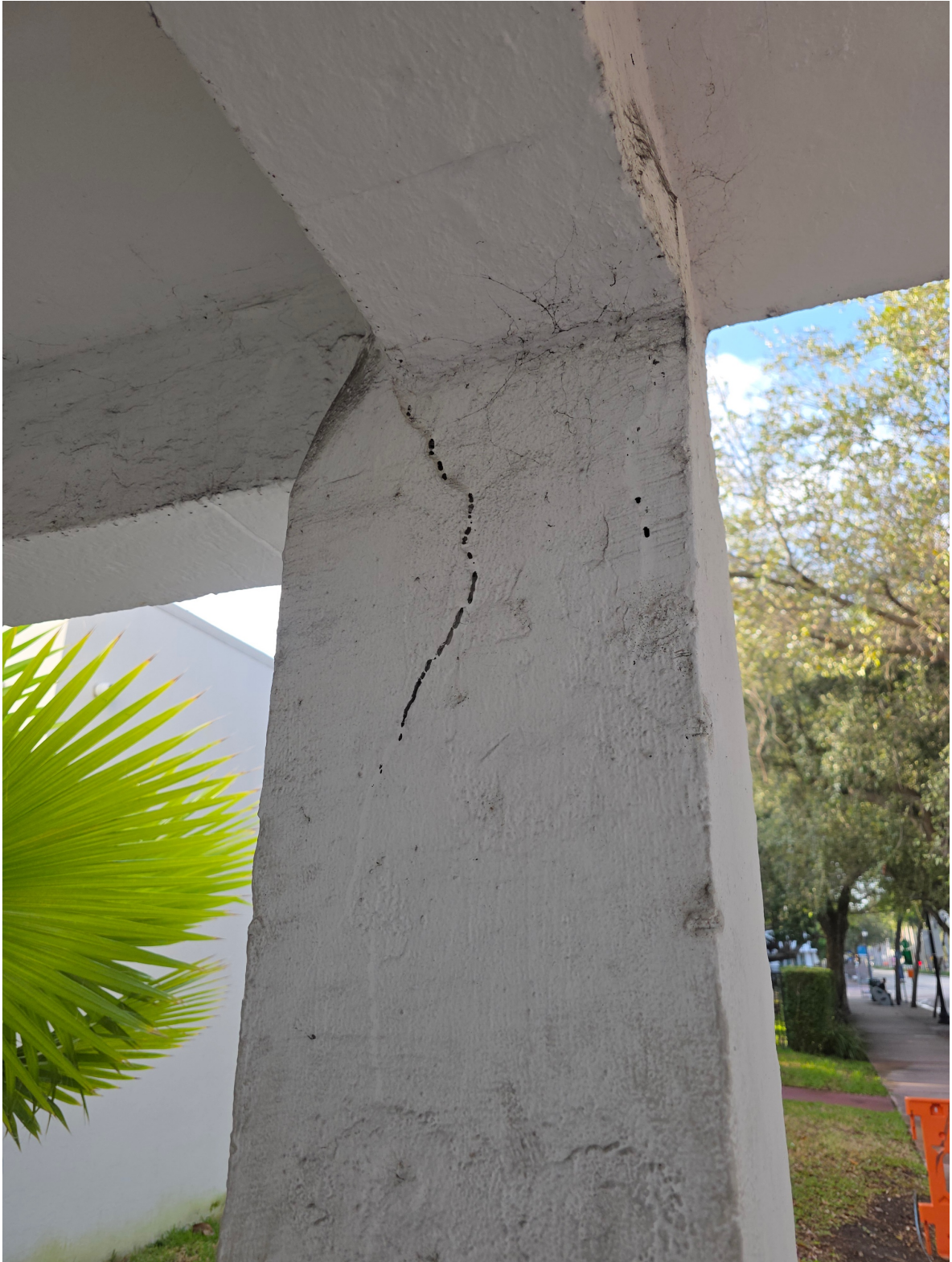
Spall and delaminated stucco and concrete present
