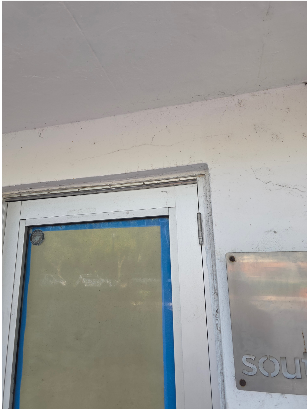
Spall and delaminated stucco and concrete present
