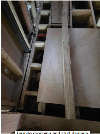
Termite dropping and stud damage
