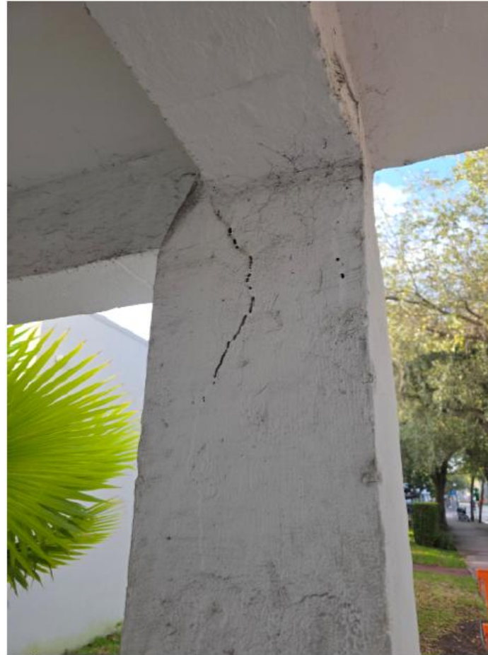
Spall and delaminated stucco and concrete present
