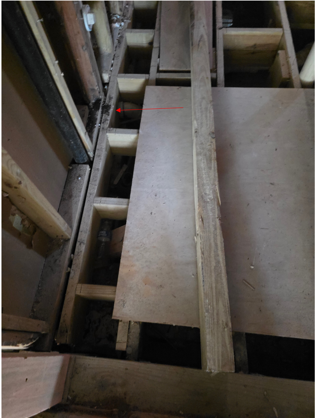
Termite dropping and stud damage
