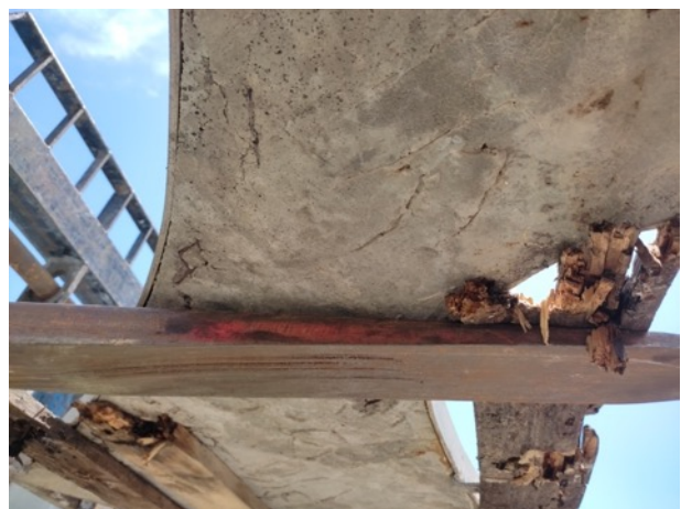
Detail of cracks, distinguishing marks and exposed wire mesh on the back of panel #18 during relocation.
