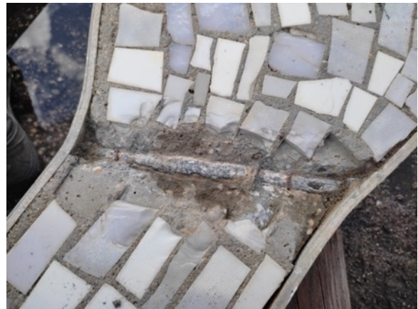
Detail of excavated aluminum tube showing internal corroded ferrous bar, and corroded wires (supposedly attached to mesh) at panel #4.
