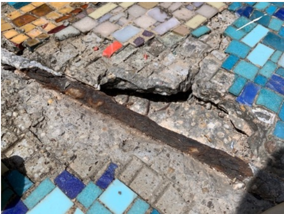
Detail of exposed aluminum tube, corroded ferrous bar, corroded wire mesh, and large cavity at panel #1.
