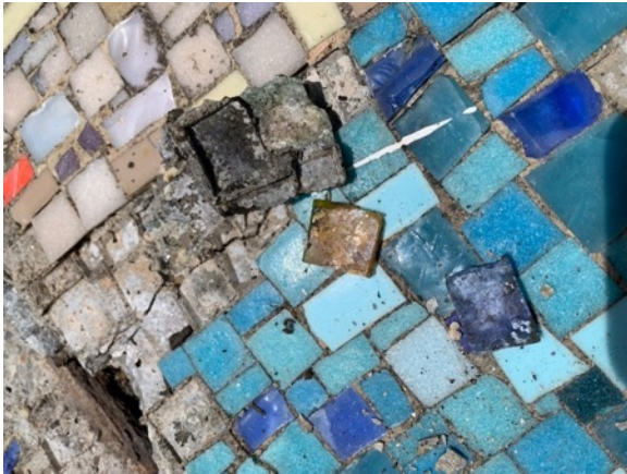
Detail of panel #1, showing dislodged tiles with bio growth visible on both the backs of the tiles as well as on the bedding mortar over which they sat.
