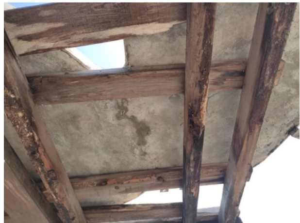
Detail of water infiltration at crack on the back of panel #17 during relocation.
