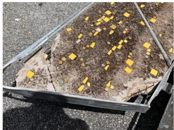
Detail of exposed aluminum tube, cracks, concrete loss and exposed corroded wire mesh on 'ground' panel during excavation.
