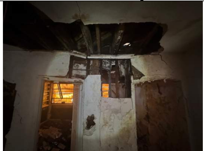
Wood Damage and failure
