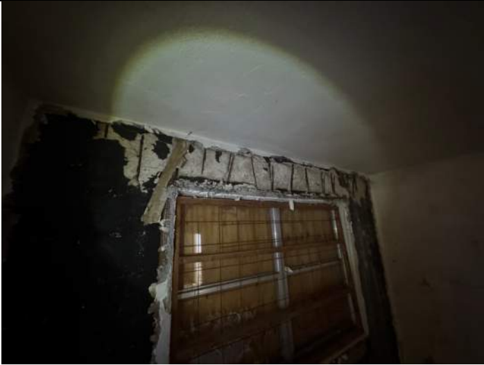
Concrete beam spalling and rebar corrosion
