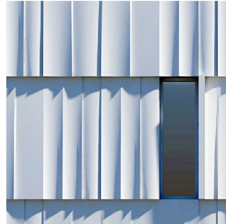
SCULPTURAL PRECAST PANELS at the second and third floors of new addition
