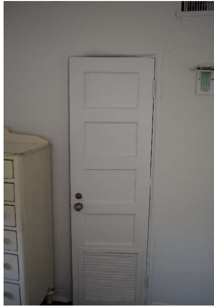
Figure 38. Interior closet door at Bedroom 4, May 2021.
