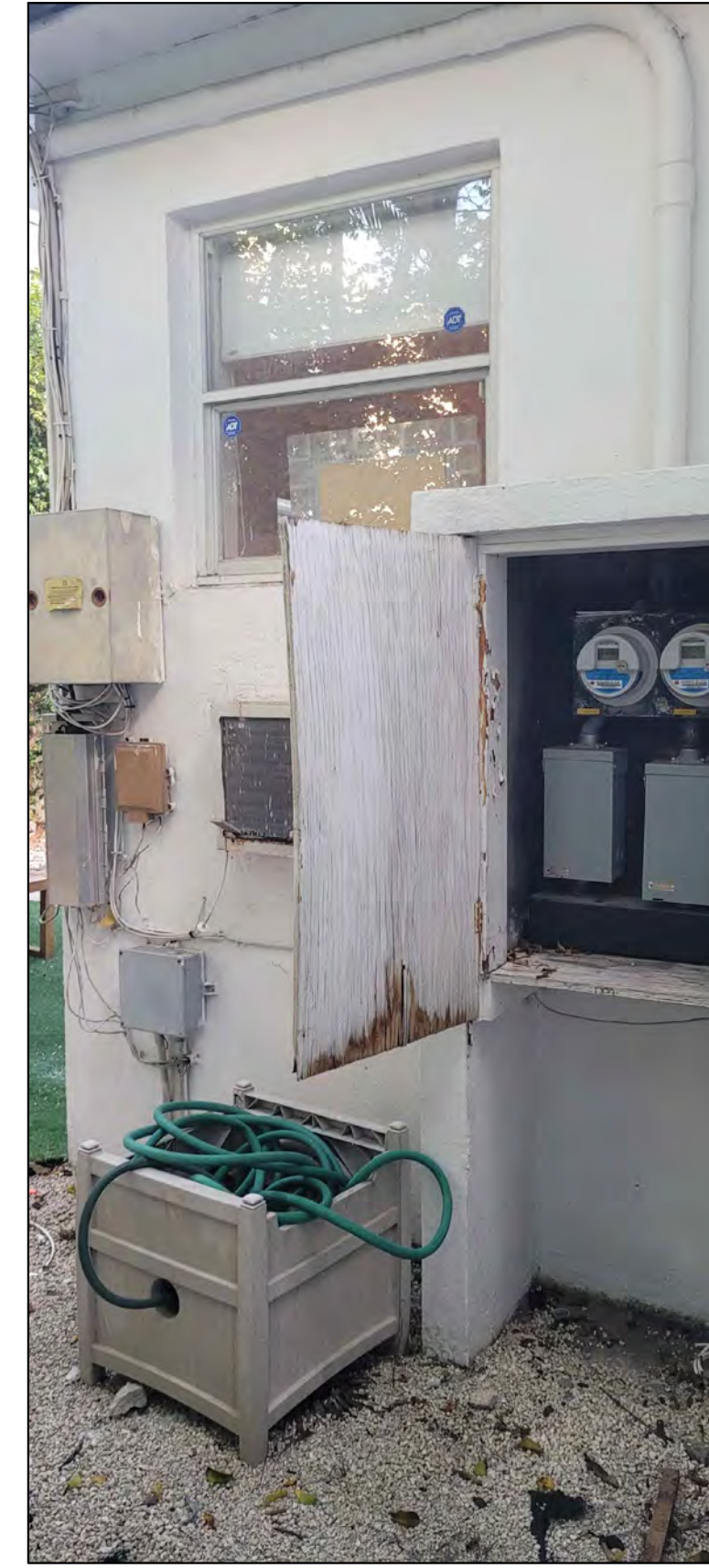
UTILITY CONNECTIONS AT NORTH (REAR) FACADE TO BE DEMOLISHED
