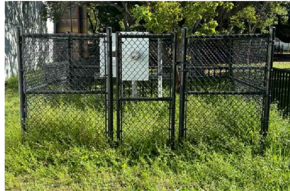
20. ELECTRICAL PANELS IN THE MIDDLE OF FPL STAGING AREA
