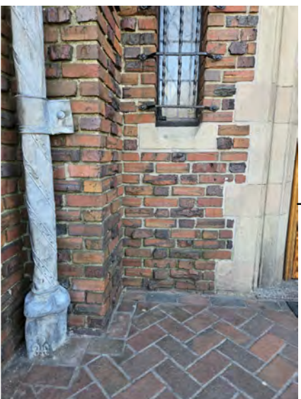
PRECAST STONE MOULDING AND BRICK
