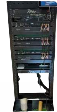
SMART HOME SYSTEM PANELS
