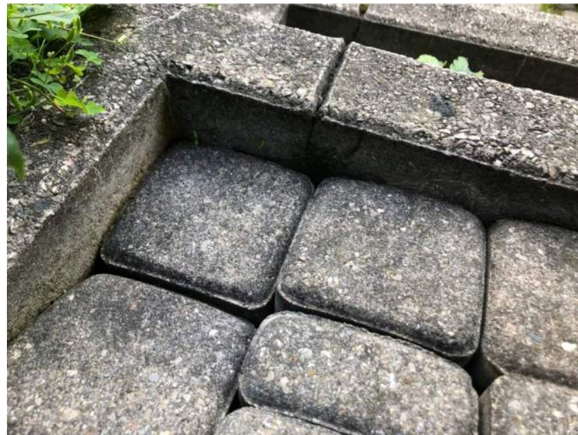
PAVER SETTLEMENT PHOTO
