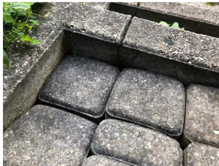
PAVER SETTLEMENT PHOTO
