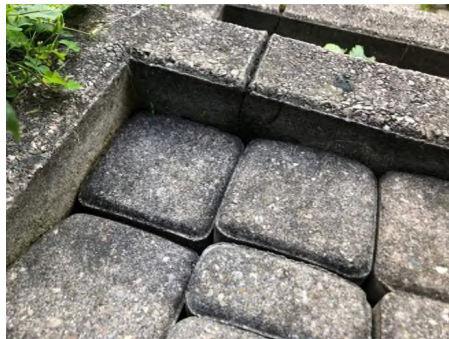
PAVER SETTLEMENT PHOTO
