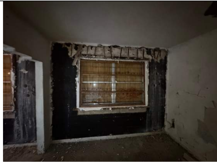
2 nd floor concrete beam damage
