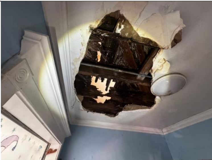
2 nd floor wood failure
