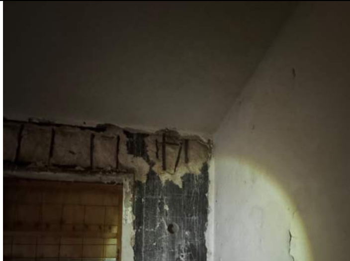
Critical Linear Crack concrete grade beam
