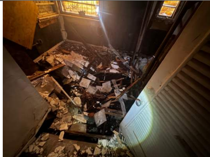
1 st floor wood failure
