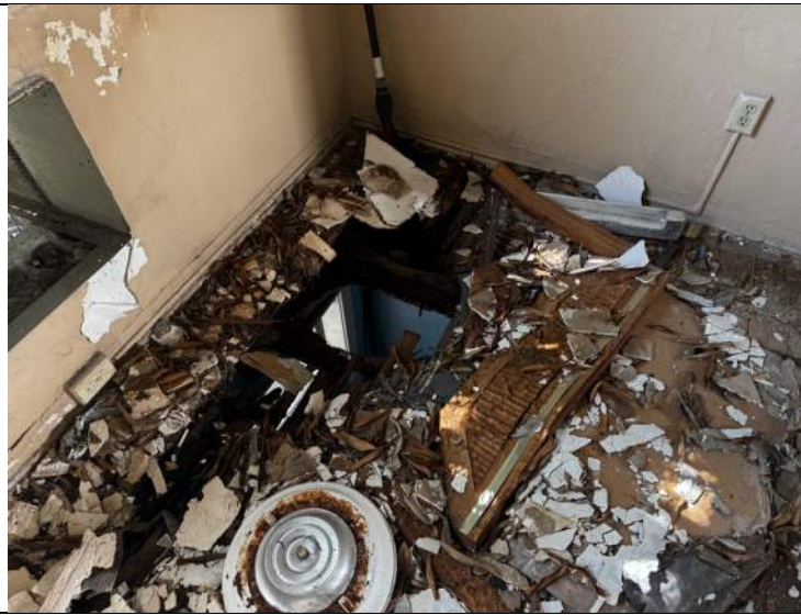
2 nd floor damage
