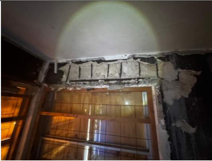
Concrete beam spalling and rebar corrosion
