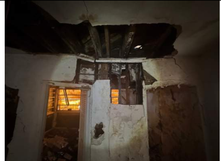
Wood Damage and failure
