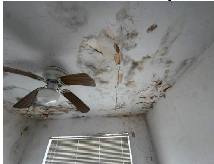
Roof moisture penetration damage
