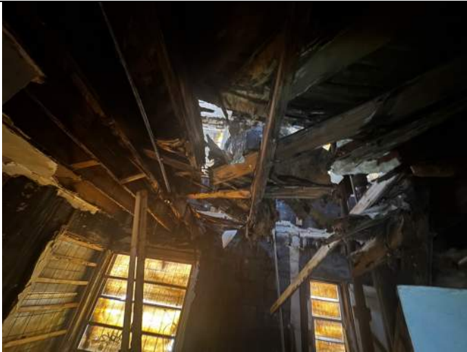
2 nd floor wood failure
