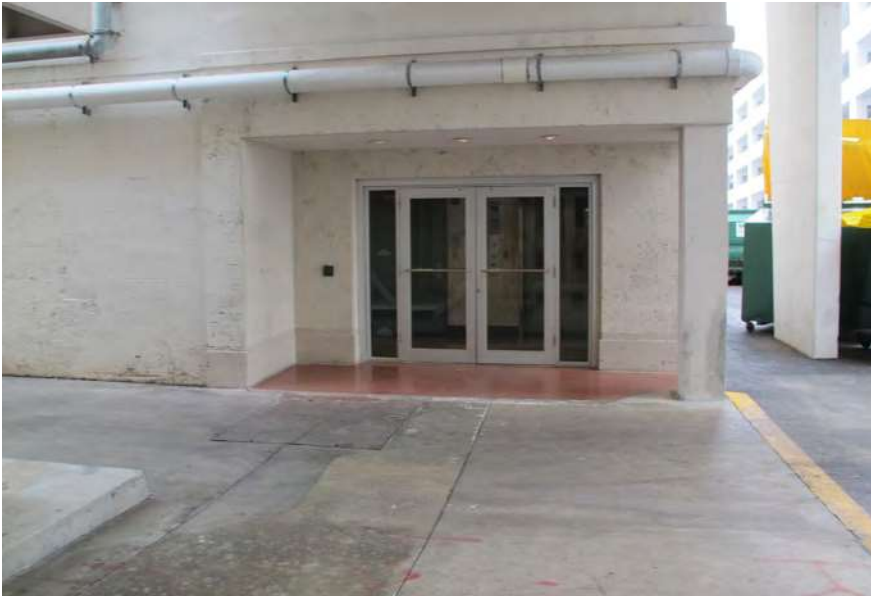
Rear (west) entrance to the Washington Avenue Annex Building. View looking South.
