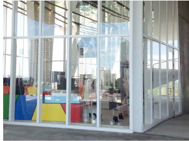
GL-01: CLEAR VISION, LAMINATED STOREFRONT GLASS MTL-01: PAINTED, EXTRUDED ALUMINUM, STOREFRONT SYSTEM
