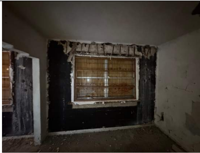
2 nd floor concrete beam damage
