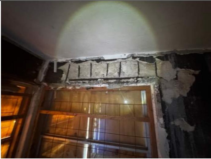
Concrete beam spalling and rebar corrosion
