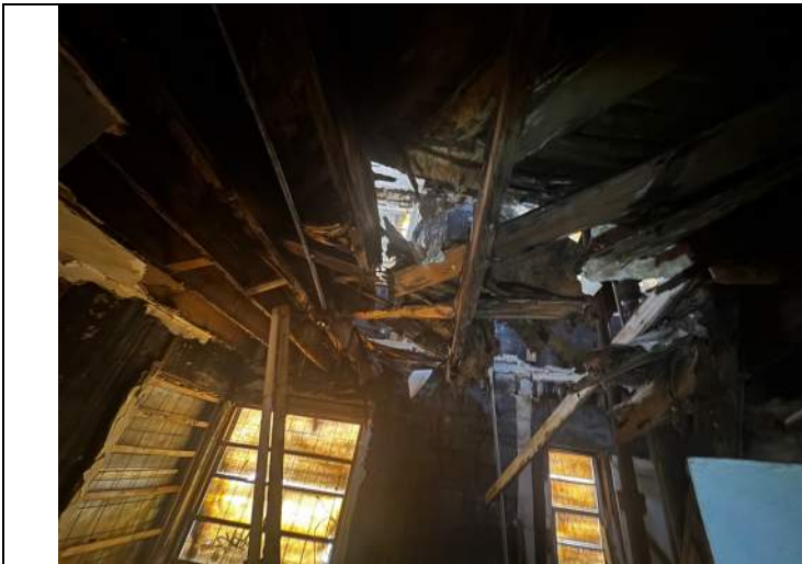
2 nd floor wood failure
