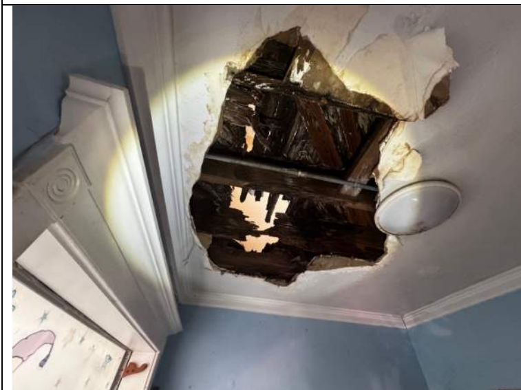
2 nd floor wood failure
