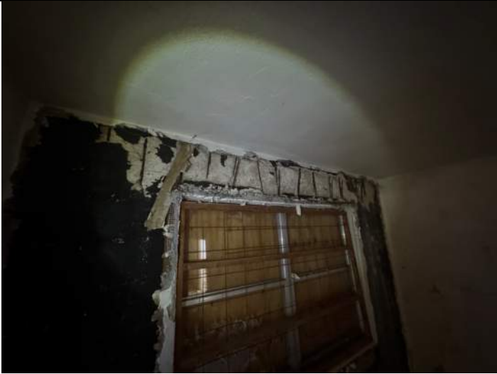
Concrete beam spalling and rebar corrosion
