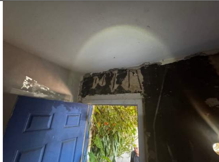
Concrete beam spalling and rebar corrosion
