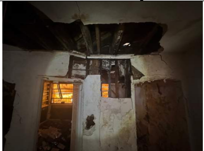
Wood Damage and failure
