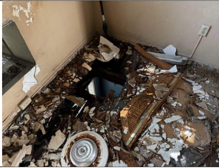
2 nd floor damage
