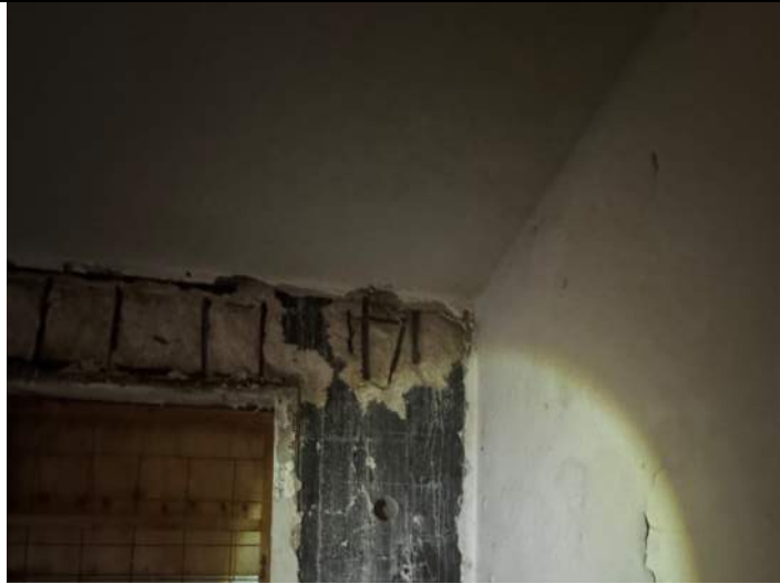
Critical Linear Crack concrete grade beam
