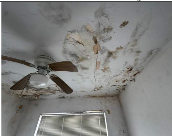
Roof moisture penetration damage
