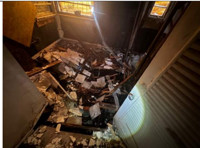
1 st floor wood failure
