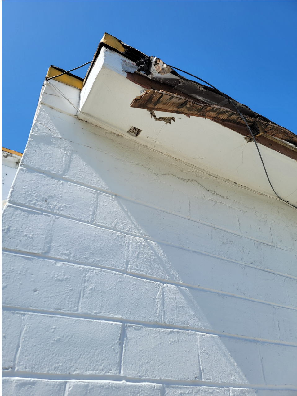
Rotted wood present on fascia
