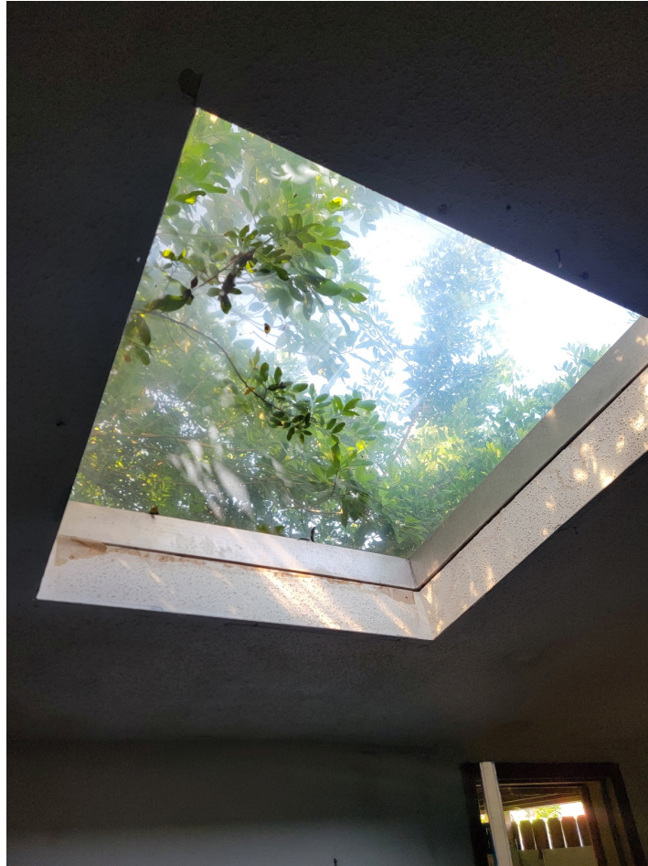
Skylights present show water intrusion.
