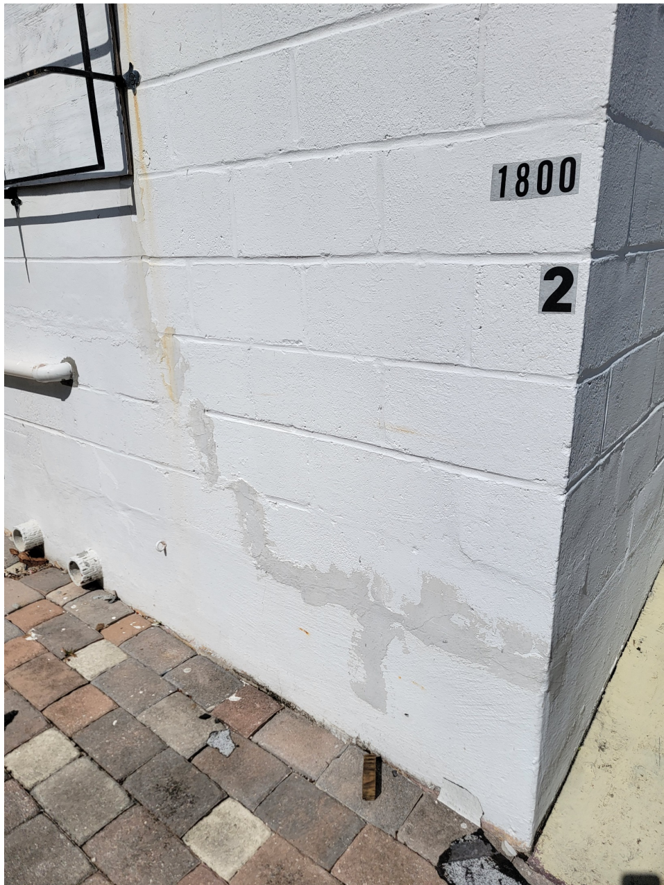
Cracks noted leading to foundations
