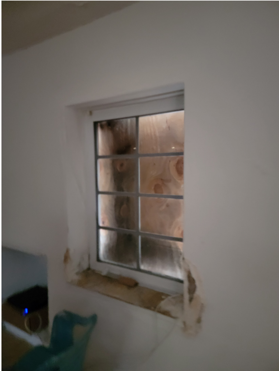
Water intrusion thru windows
