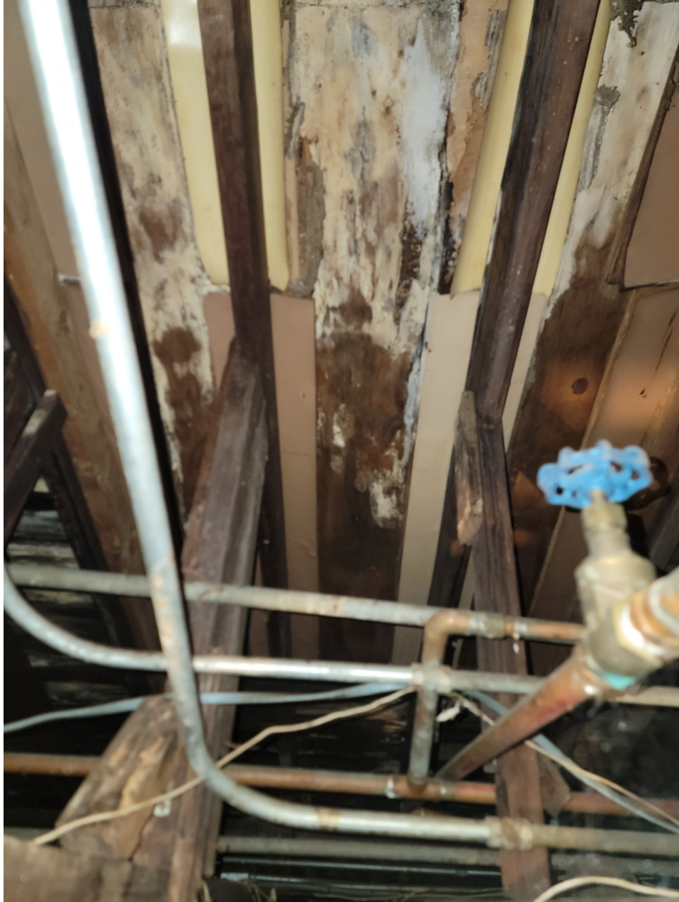
Water intrusion noticed coming from roof
