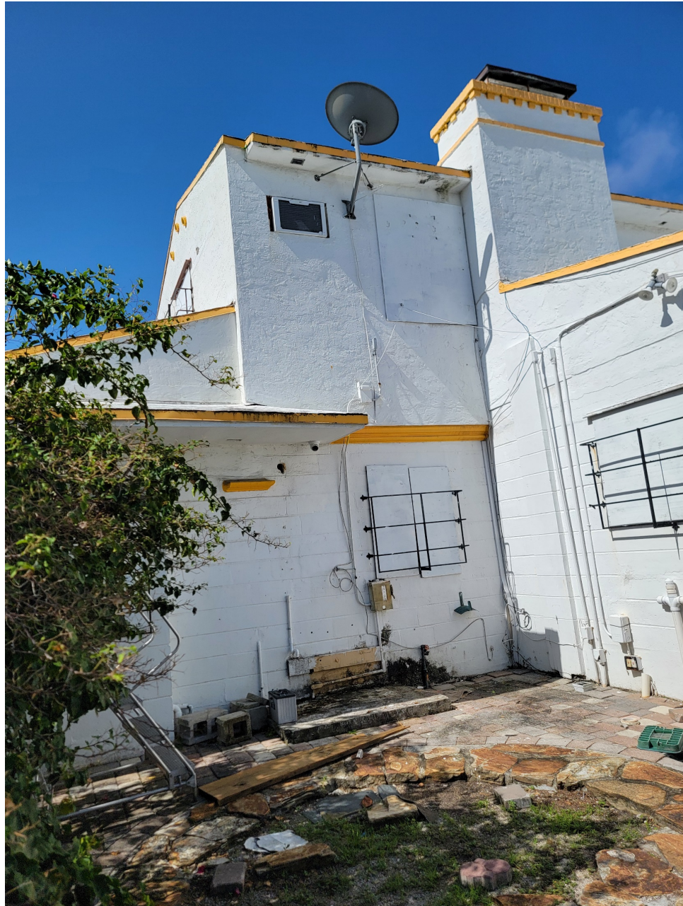
Spall and delaminated stucco present
