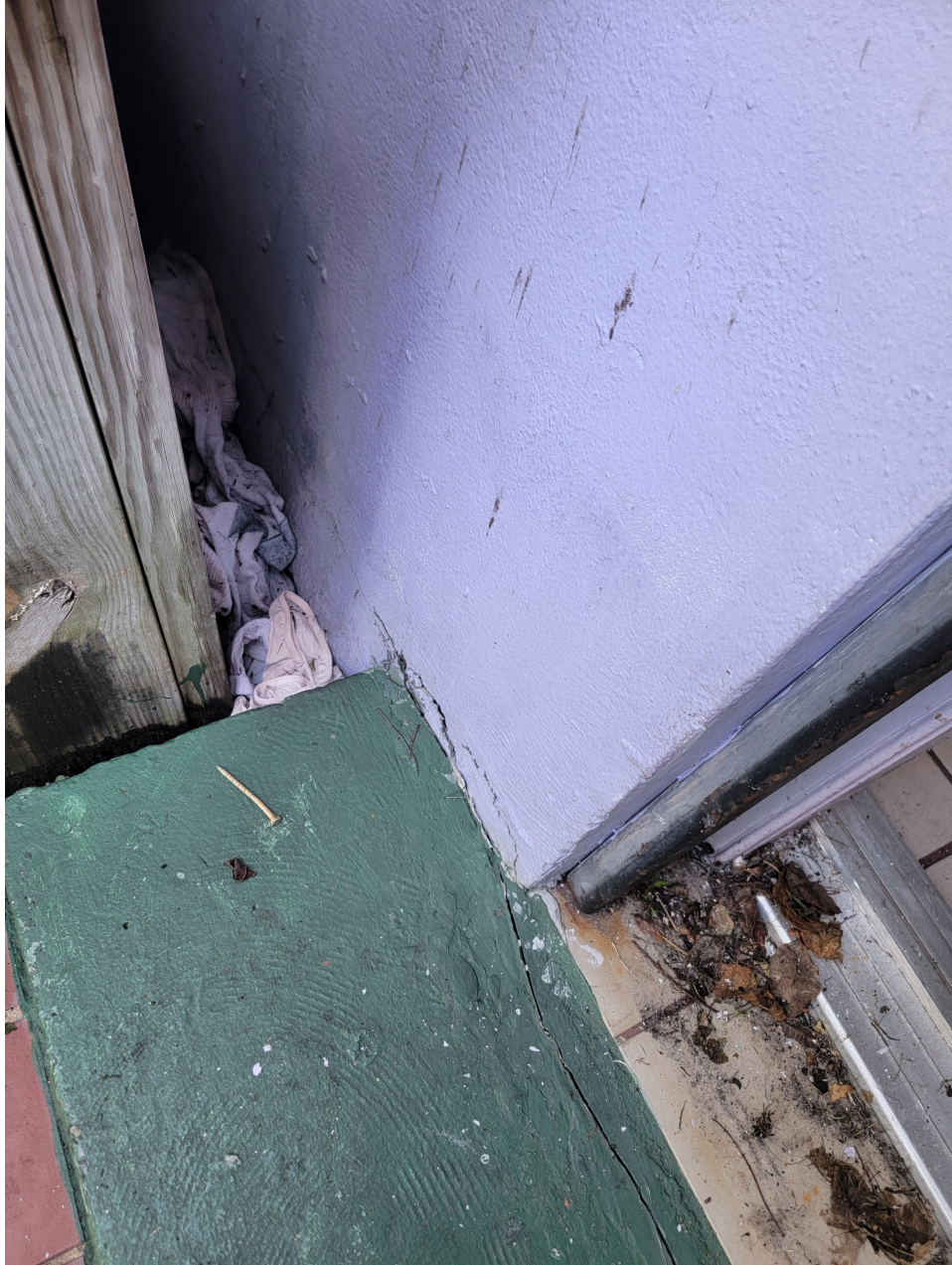
Deflections noticed on foundations
