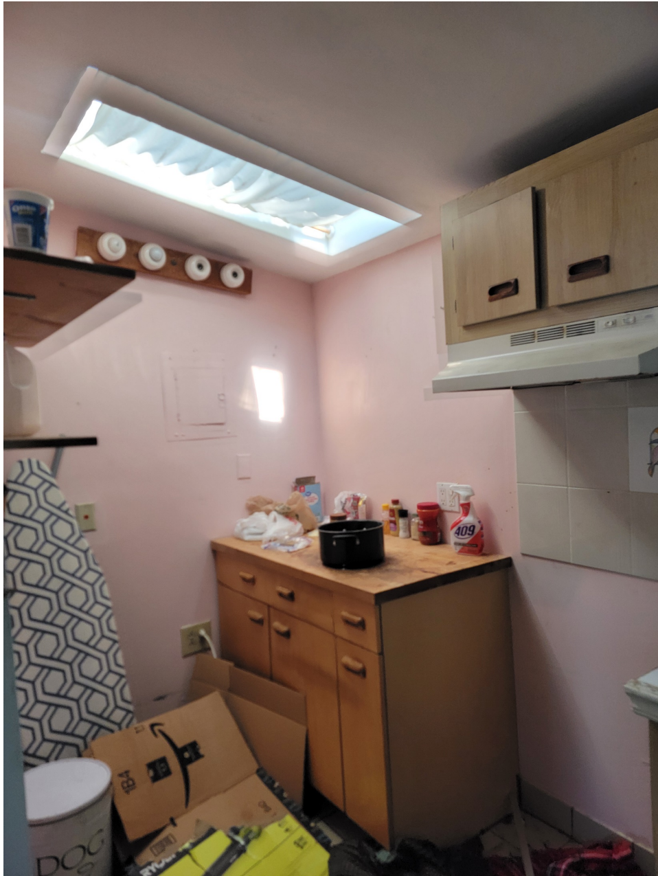
Skylights failure noticed
