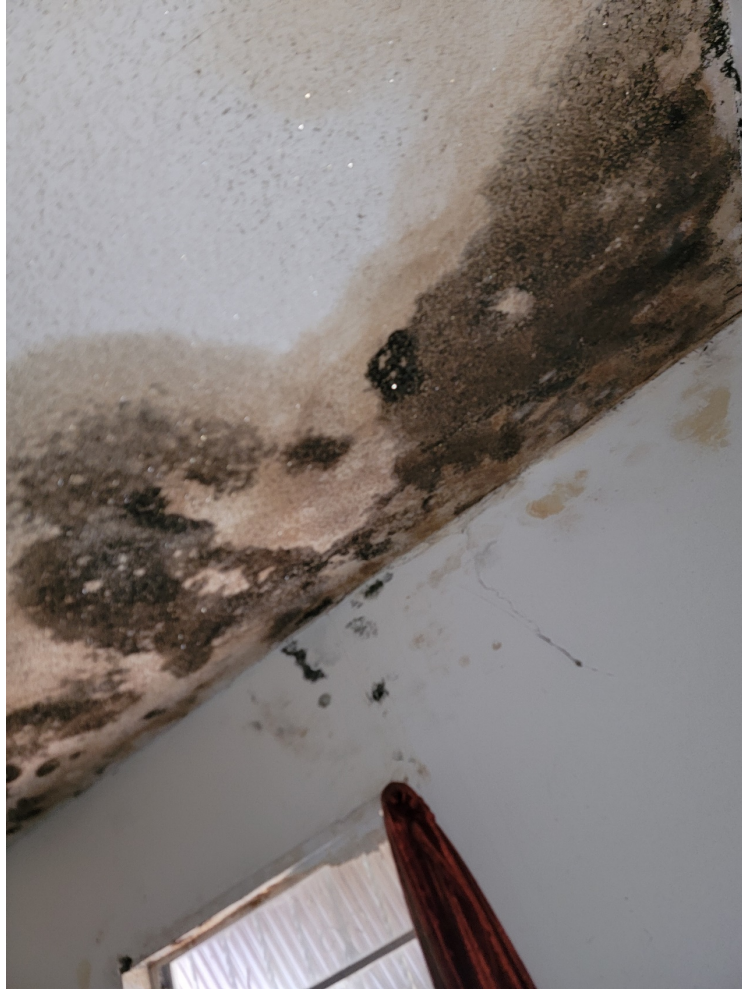
Mold and water intrusion is present
