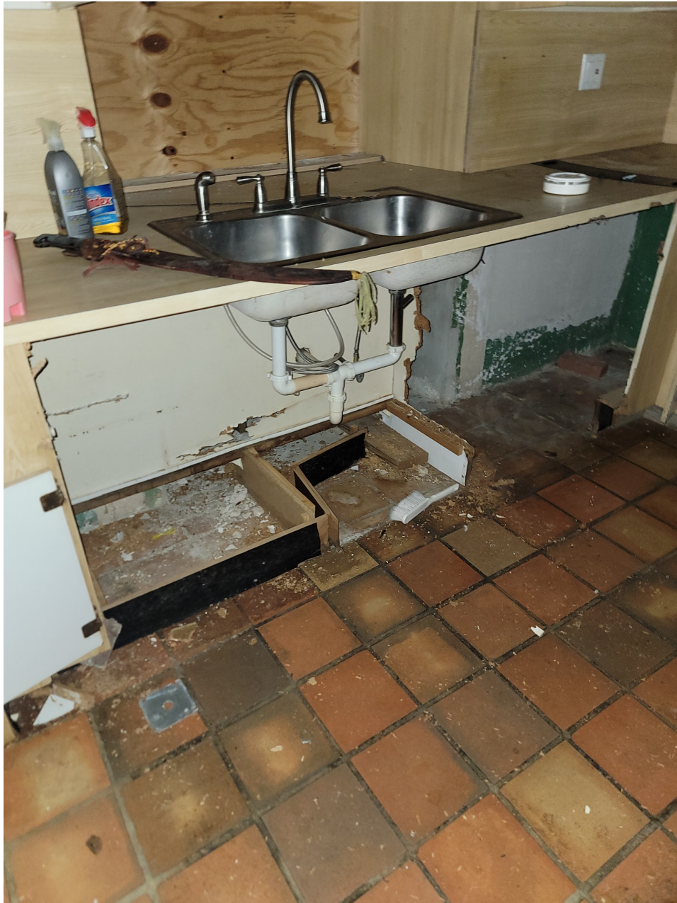
Water intrusion damages noted
