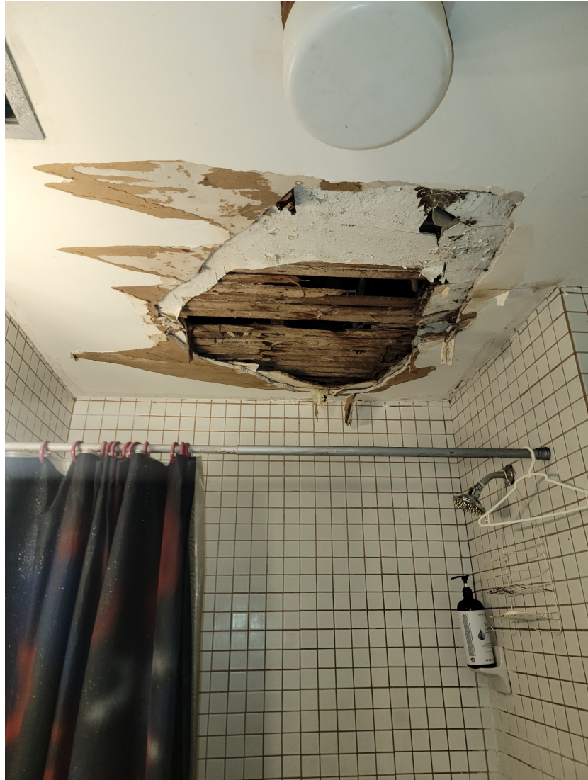
Water intrusion is present throughout the entire property
