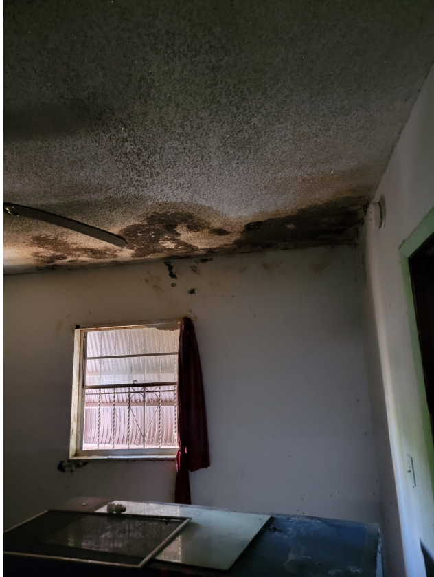
Mold is present on the interior finishes
