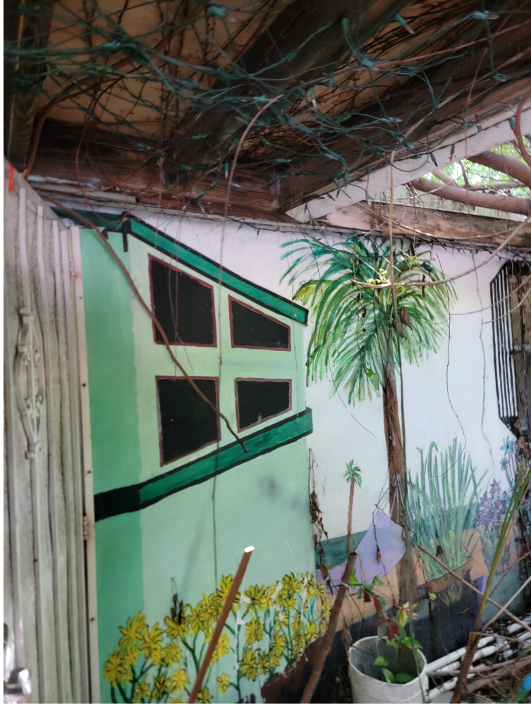
Failures noted in the exterior wood canopy
