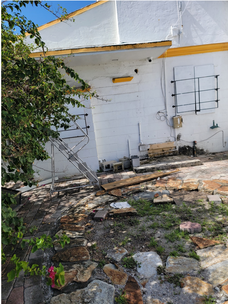
Spall and delaminated stucco present
