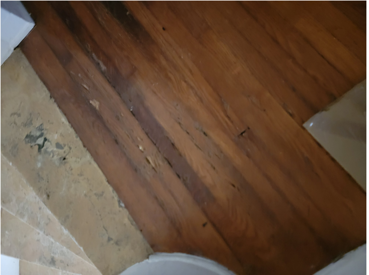
Termite damages noticed on wood floors
