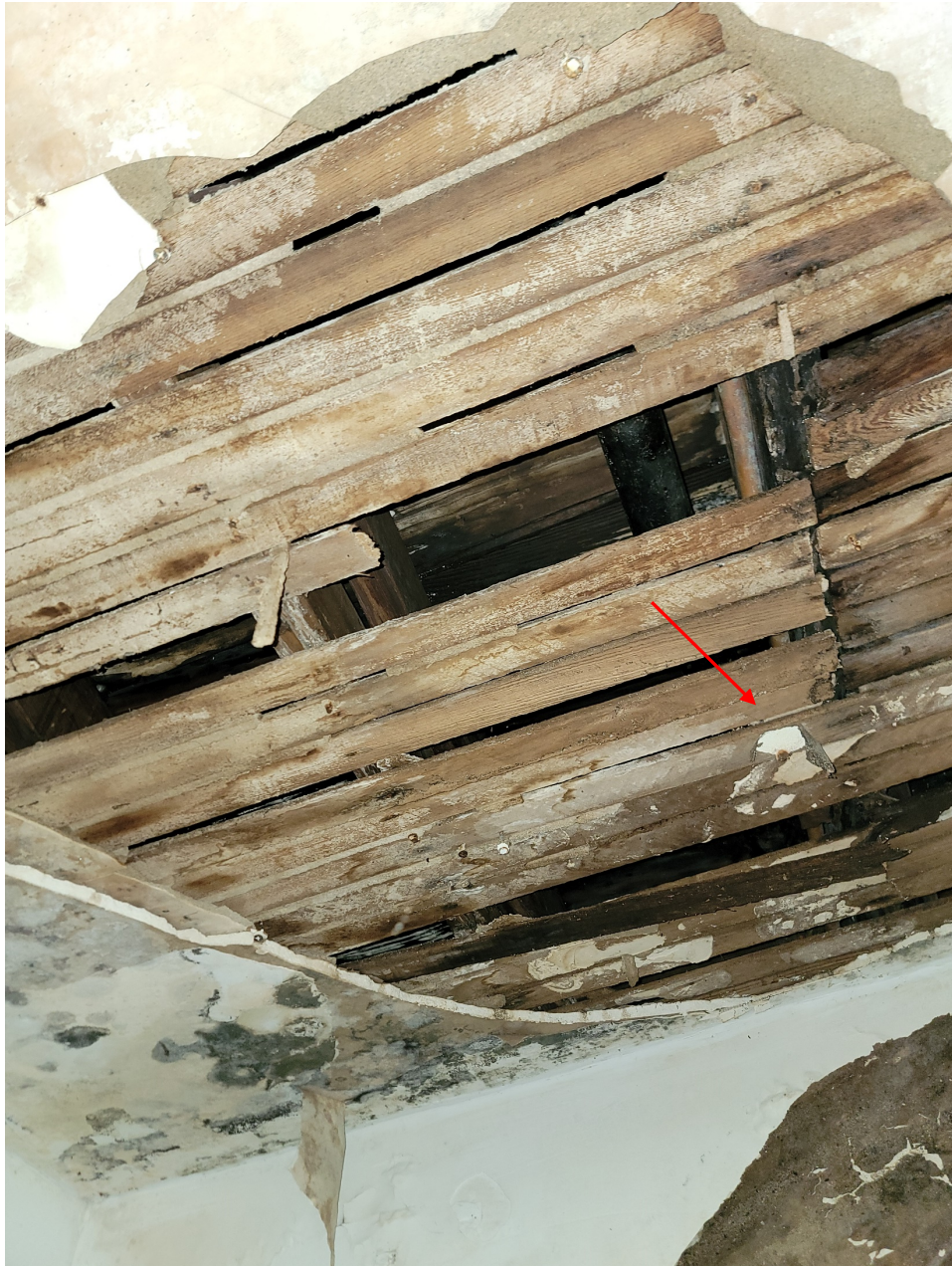
Rotted wood is noticed on the wood joist that make up the second floor of the property
