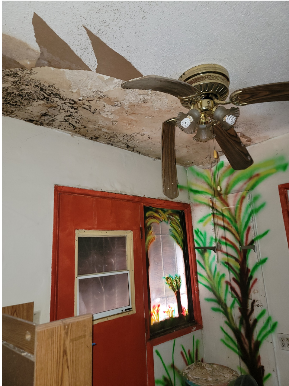
Mold present in interior finishes due to water intrusion
