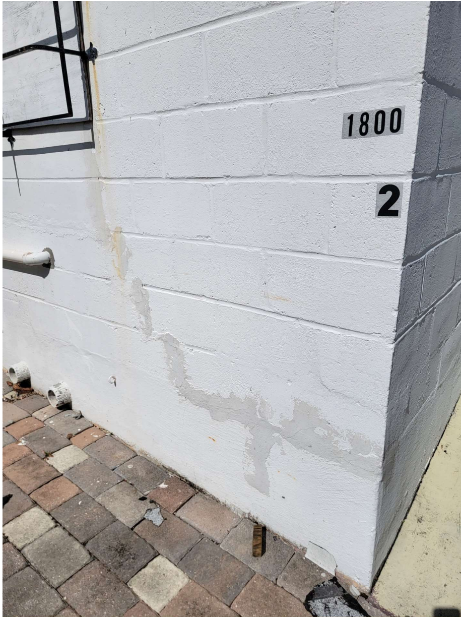
Cracks noted leading to foundations
