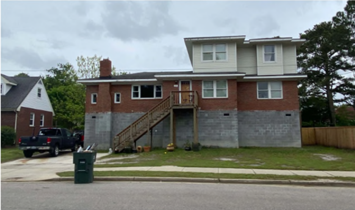
Raising a home involves lifting it off the ground and building a new higher foundation below it.
