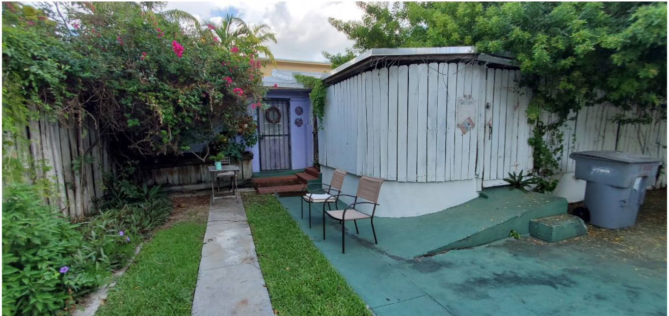
VIEW OF EXISTING DRIVEWAY SHOWING ILLEGAL ADDITION REACHING THE PROPERTY LINE AND LOCATION OF ORIGINAL GARAGE
