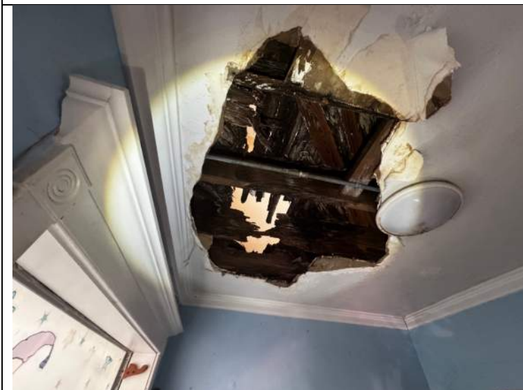
2 nd floor wood failure
