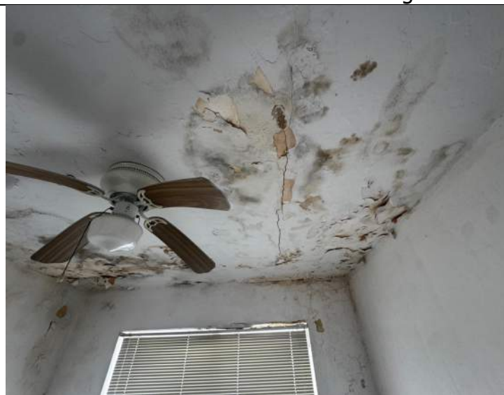
Roof moisture penetration damage
