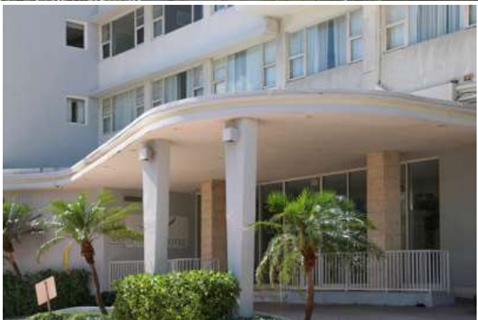
BELOW: PORTE-COCHERE WITH TWO OUTSIDE CONCRETE COLUMNS AND TWO INNER COLUMNS WHICH ARE CLAD WITH FIELDSTONE.
