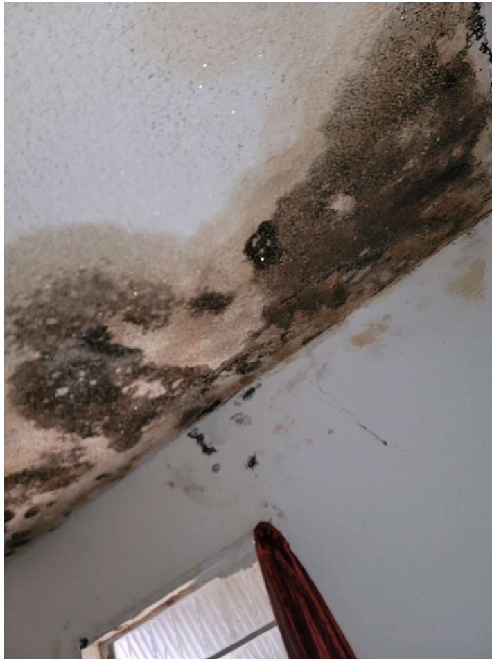
Mold and water intrusion is present
