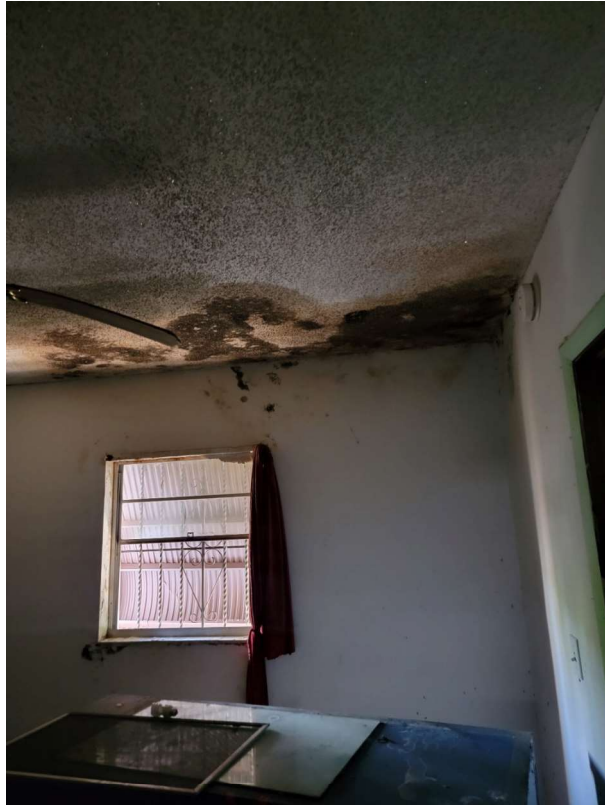
Mold is present on the interior finishes
