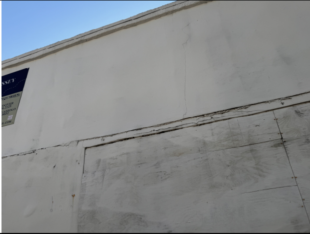
Photo 7 – Exterior stucco with cracks
