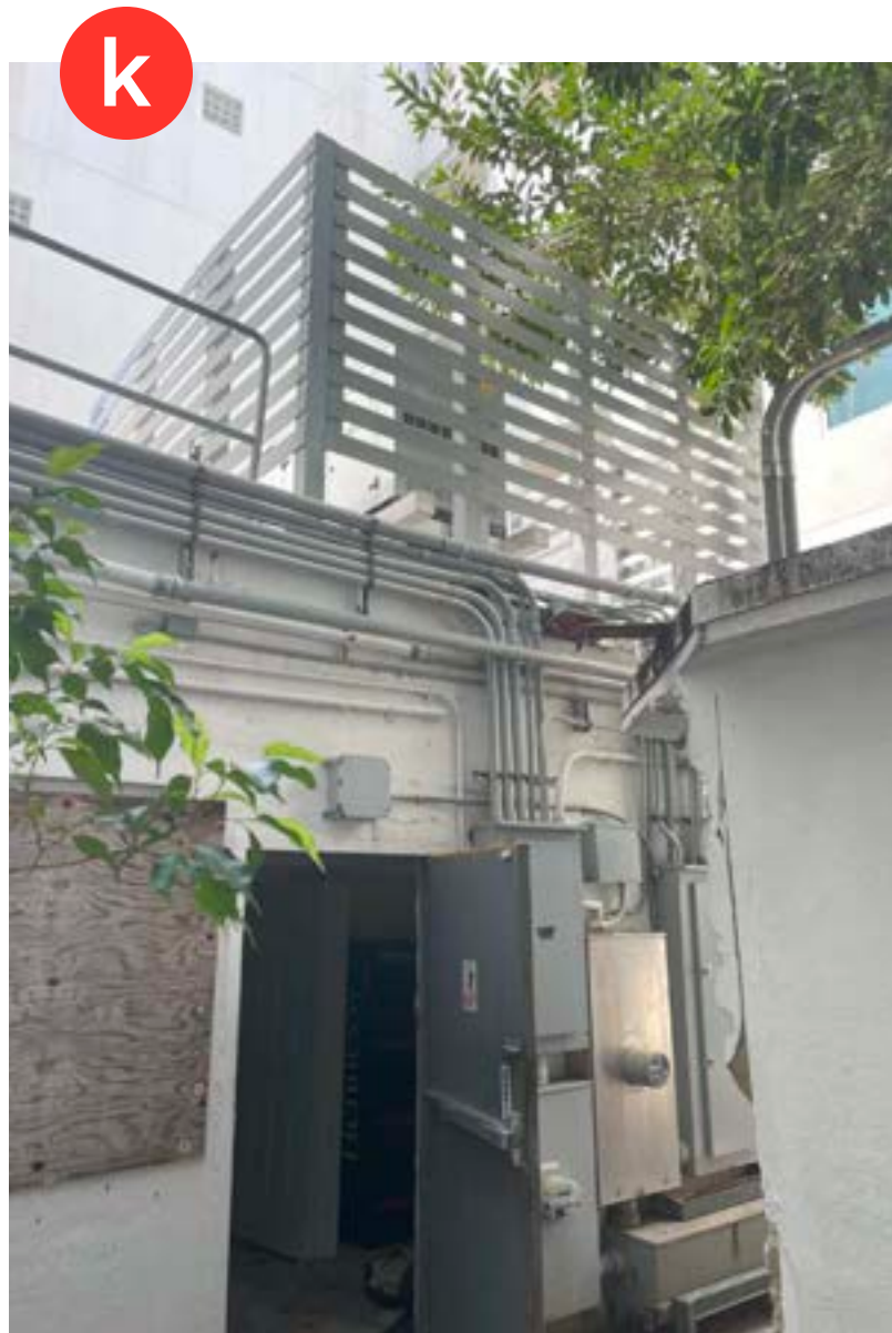
VIEW OF EXISTING MECHANICAL SCREEN ON ROOF WEST OF EXISTING STORAGE ROOM
