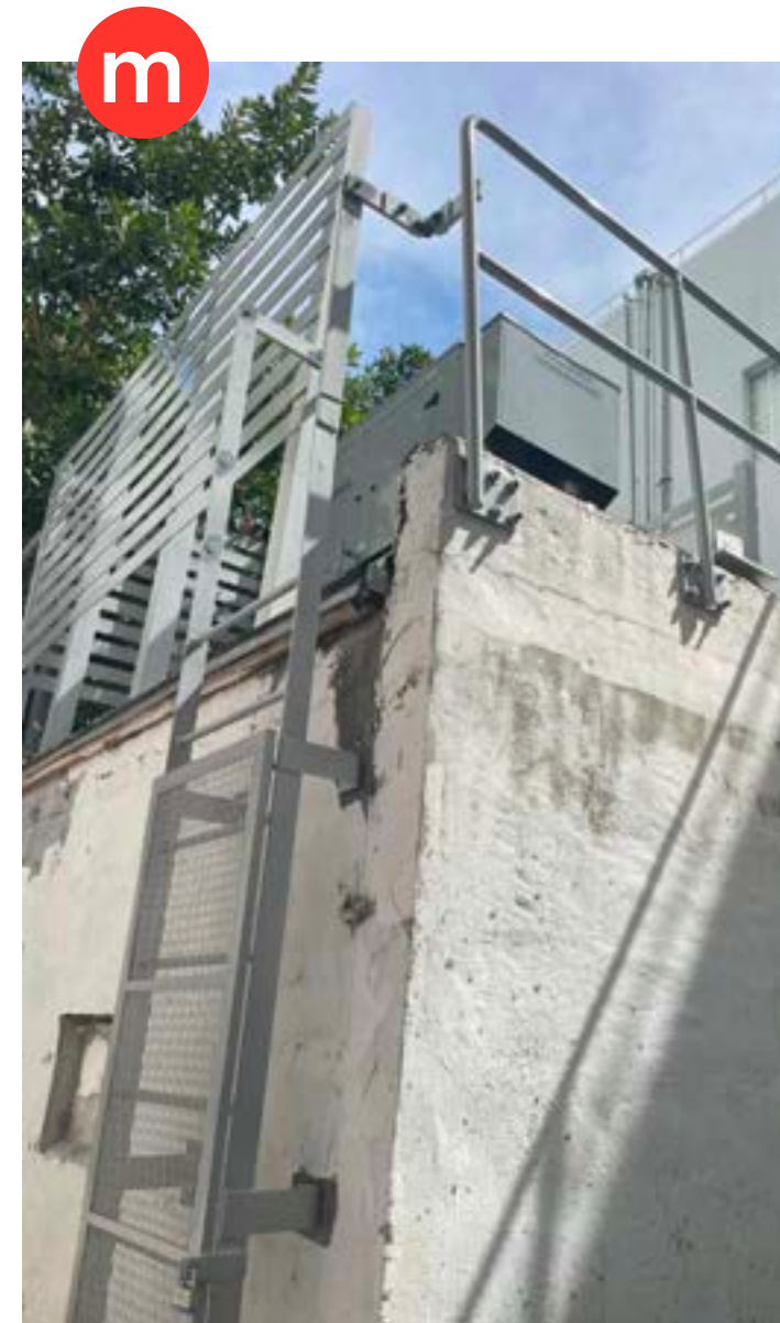
CORNER VIEW OF THE SAME MECHANICAL SCREEN
