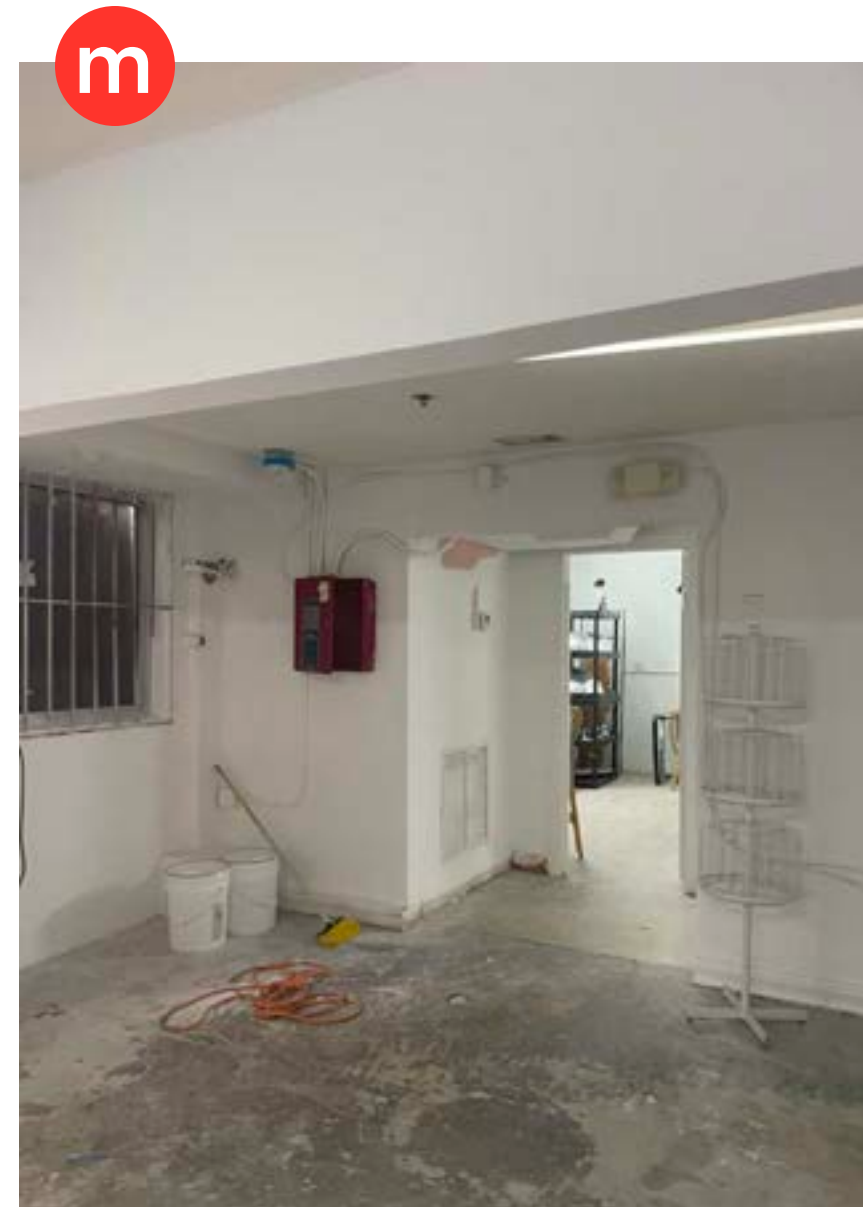
VIEW OF UNOCCUPIED TENANT SPACE (NON-CONTRIBUTING ADDITION PORTION) FACING SOUTH TOWARD PROPOSED RESTAURANT KITCHEN AREA *TERRAZZO FLOOR BEYOND INDICATES THE LINE BETWEEN DECO CONTRIBUTING STRUCTURE AND NON-CONTRIBUTING STRUCTURE)
