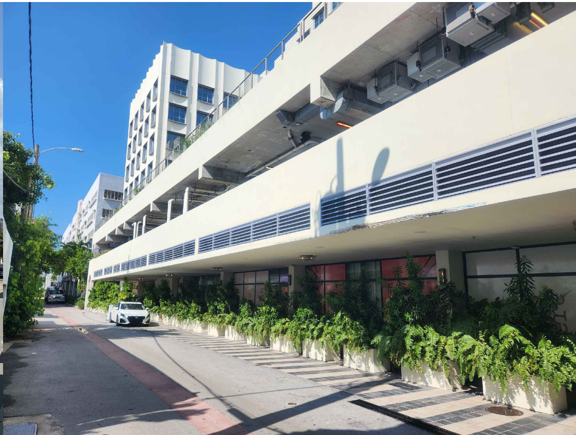
A4 VIEW FROM THE REAR OF THE BUILDING AT THE ALLEY TOWARDS 6TH STREET PHOTO TAKEN: 06-20-2023
