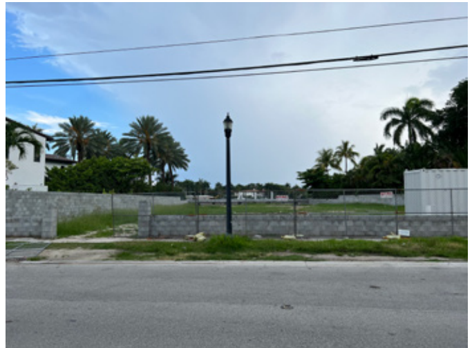
Photograph of the existing CMU site wall along the eastern site boundary
