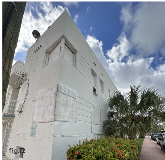
Northeast Facade | Board-up Windows | March 2024
