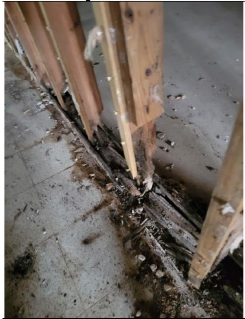
Load bearing stud walls 100% failure
