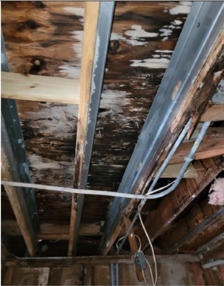
Moisture intrusion damage
