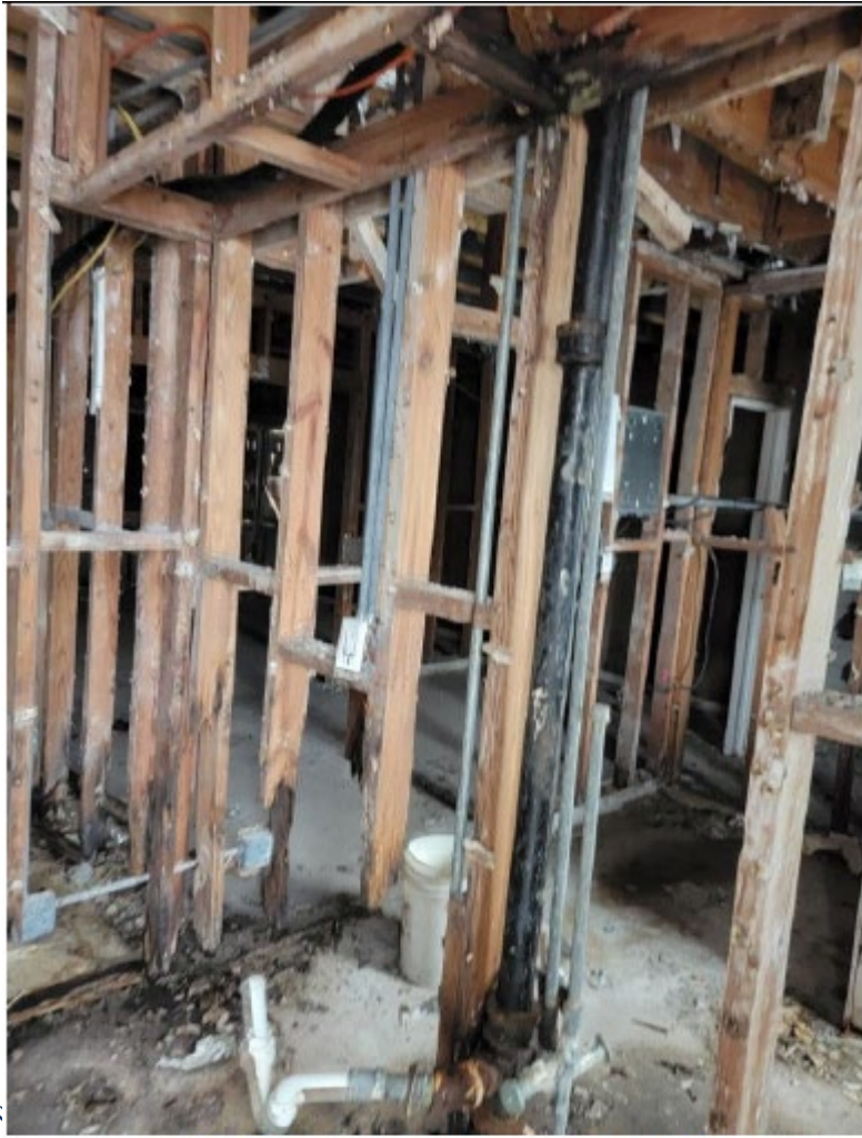
Load bearing stud walls 100% failure
