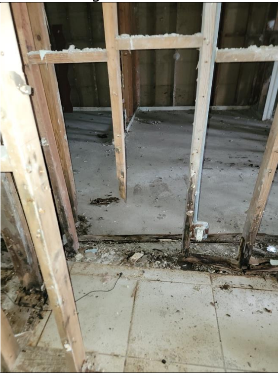
Load bearing stud walls 100% failure
