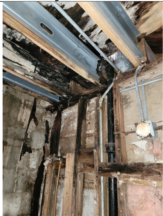
Moisture intrusion damage
