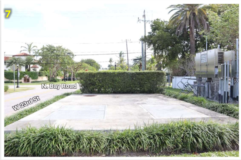
Existing Stormwater Pump Station 24 Looking East Along W 23 rd Street
