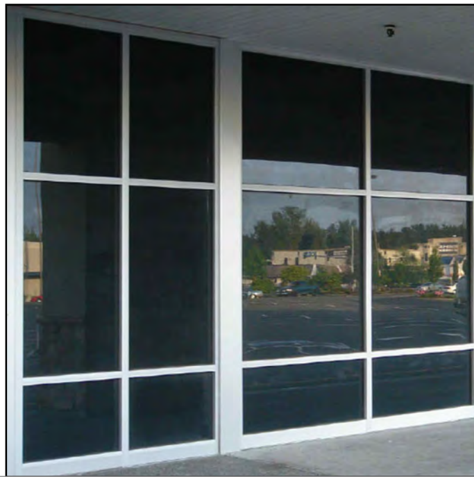
1 APPLIED OPAQUE BLACK FILM ON STOREFRONT GLAZING ELEVATION FACING THE CONDO GARDEN
