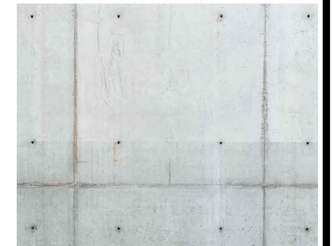
02 POOR CONCRETE FINISH
