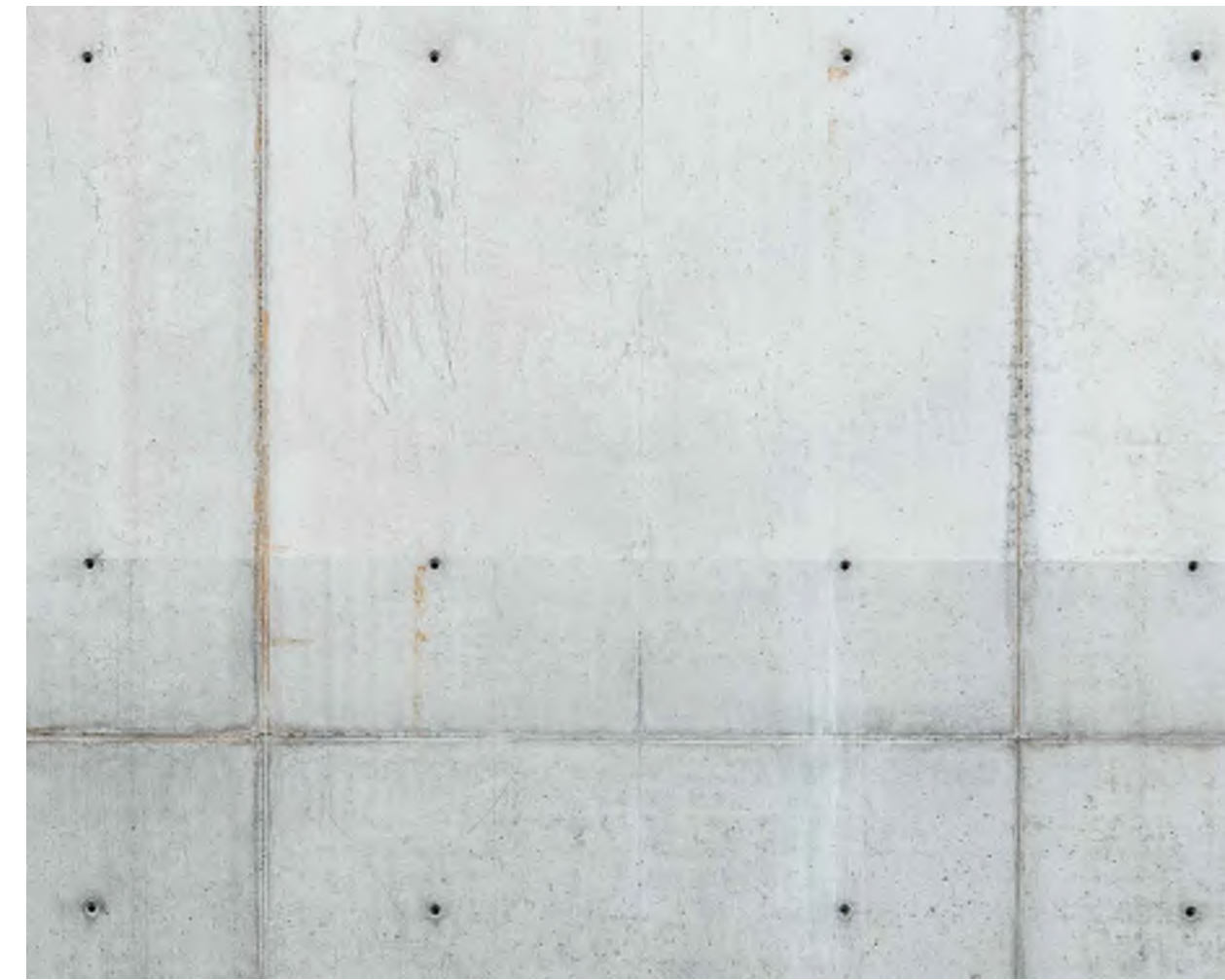
02 POOR CONCRETE FINISH
