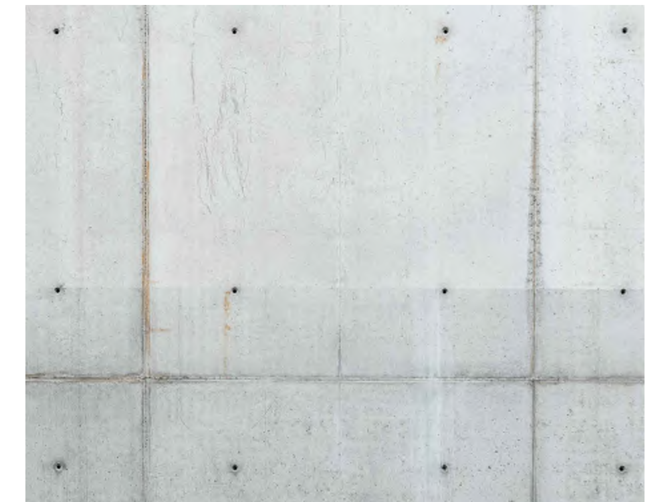
02 POOR CONCRETE FINISH
