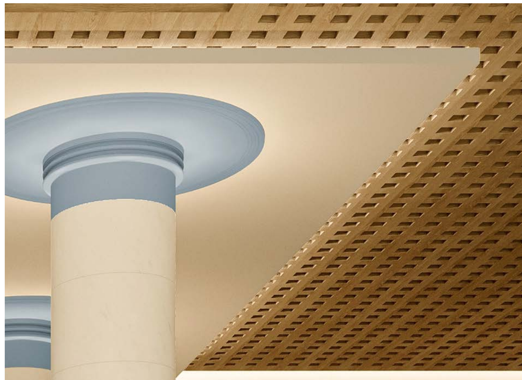
Cove lighting at drop ceiling
