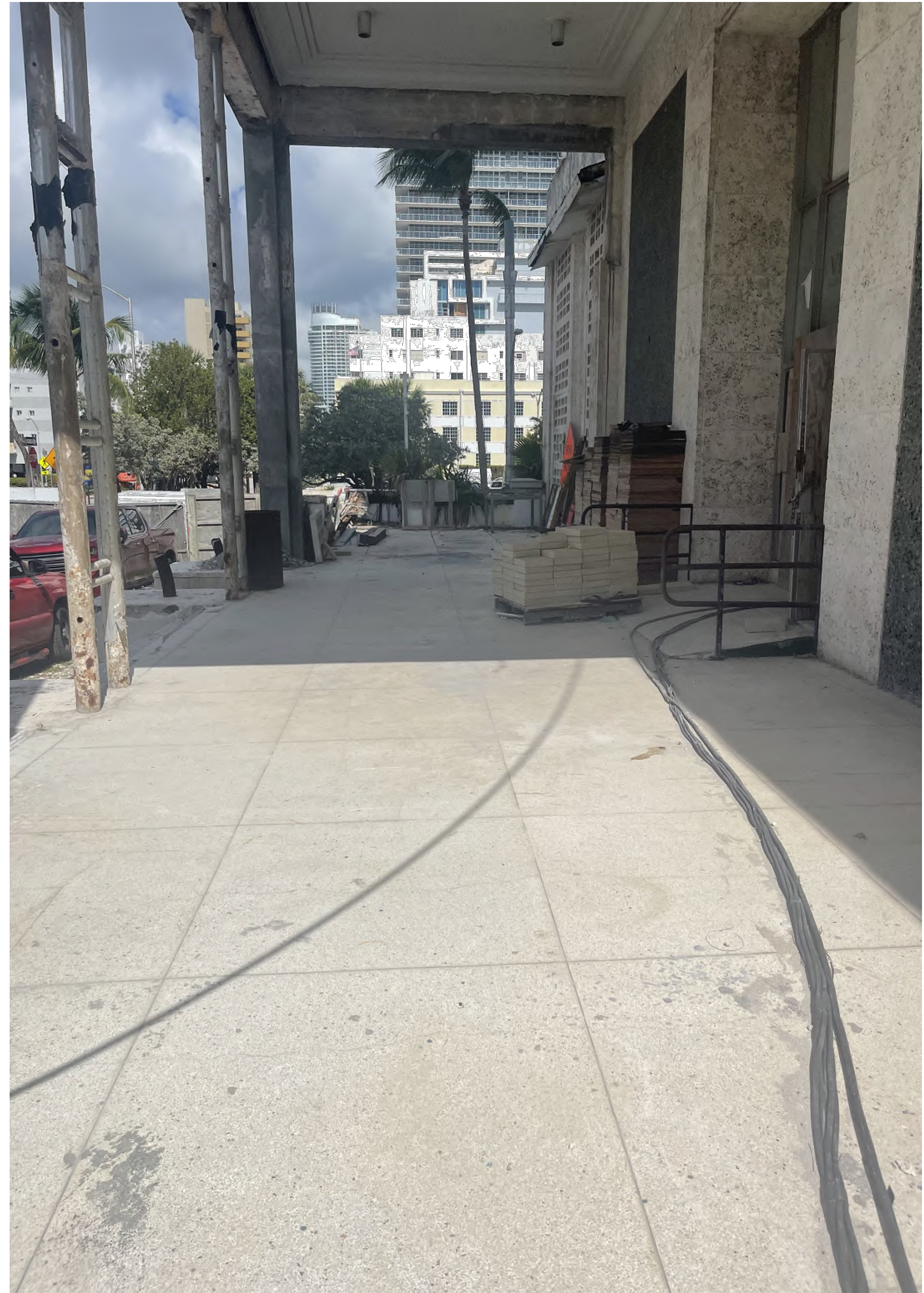
PORCHE - EXISTING CONDITIONS
